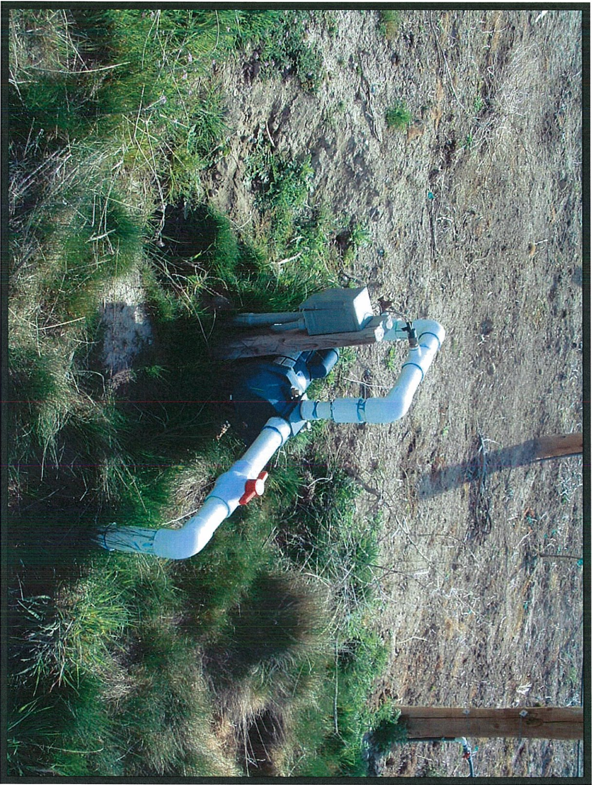
1 hp Booster Pump
