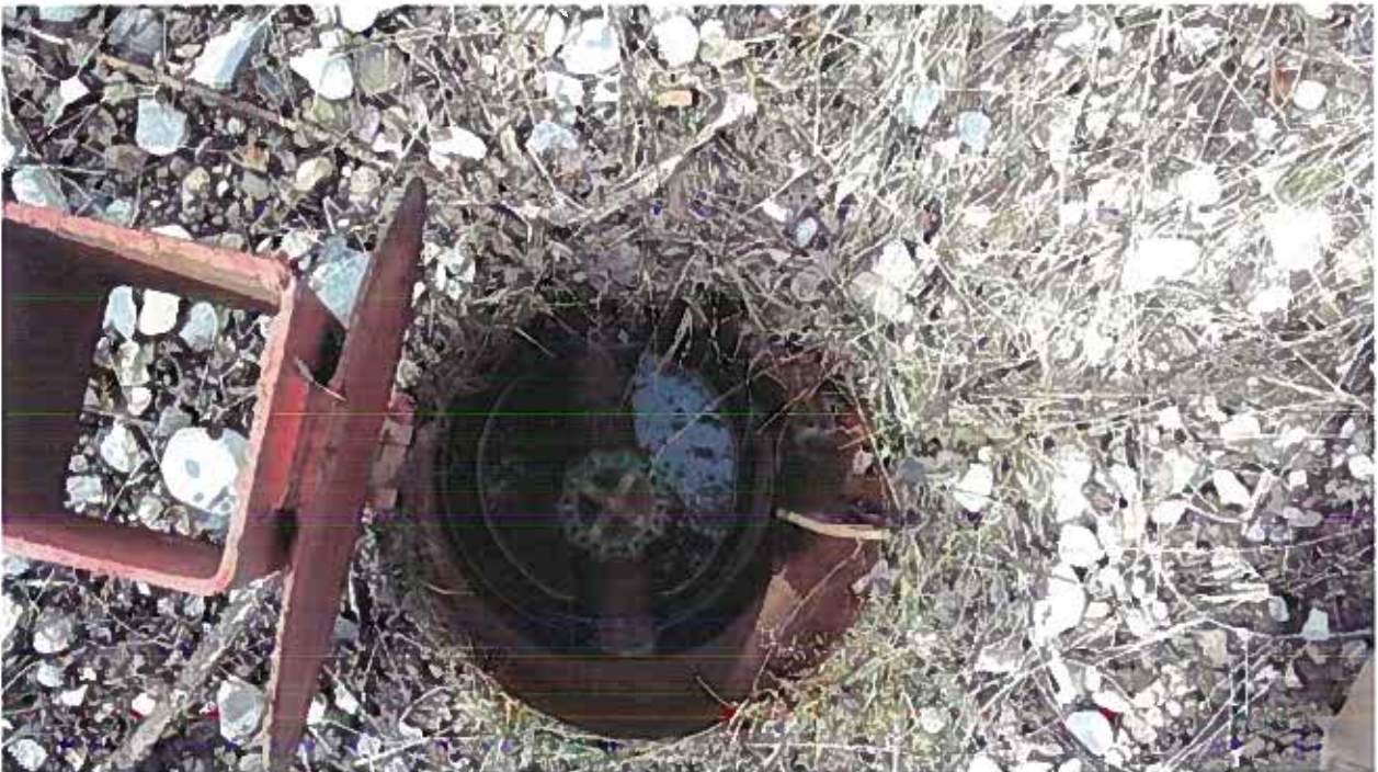
Photo 4 On/Off for system at POD
