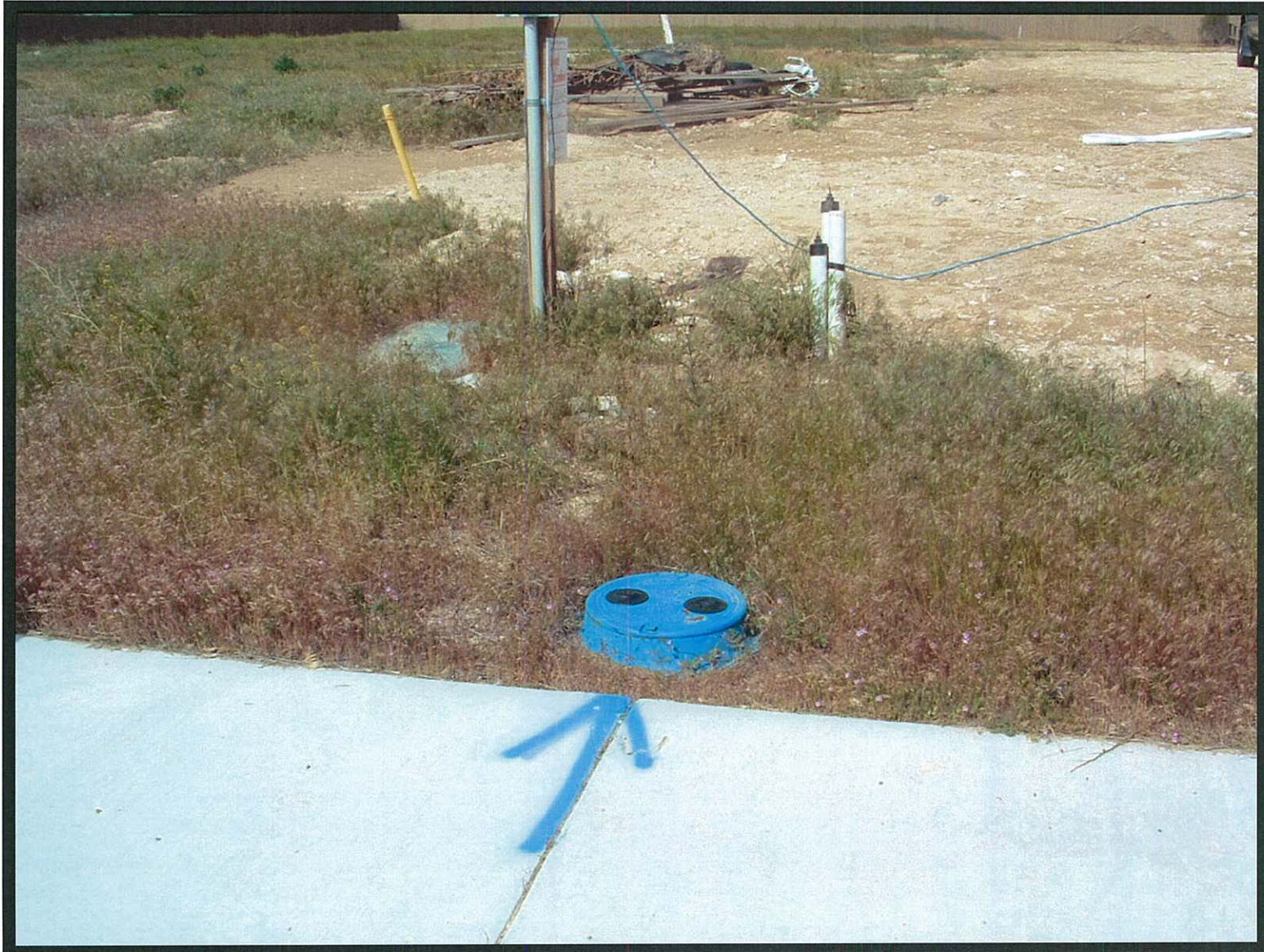
Ground Water System Stub, Lot 17, Block 1
