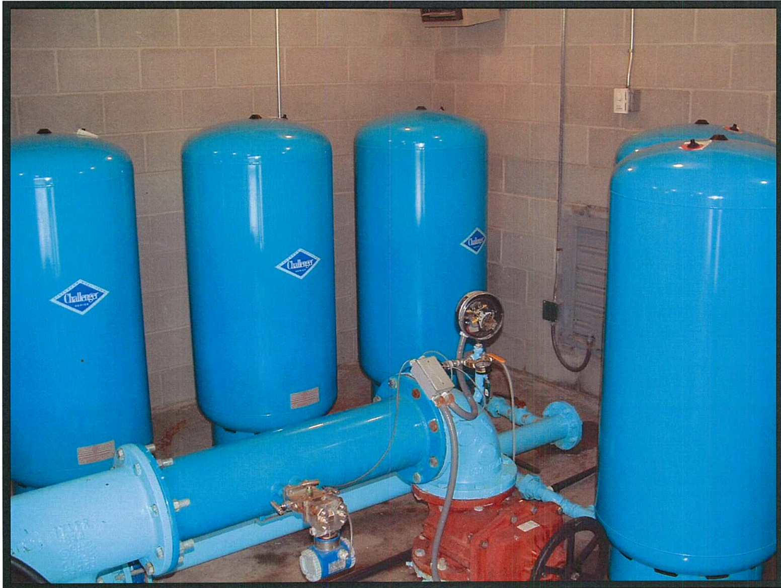
Fire Protection Flowmeter and Hydropneumatic Tanks
