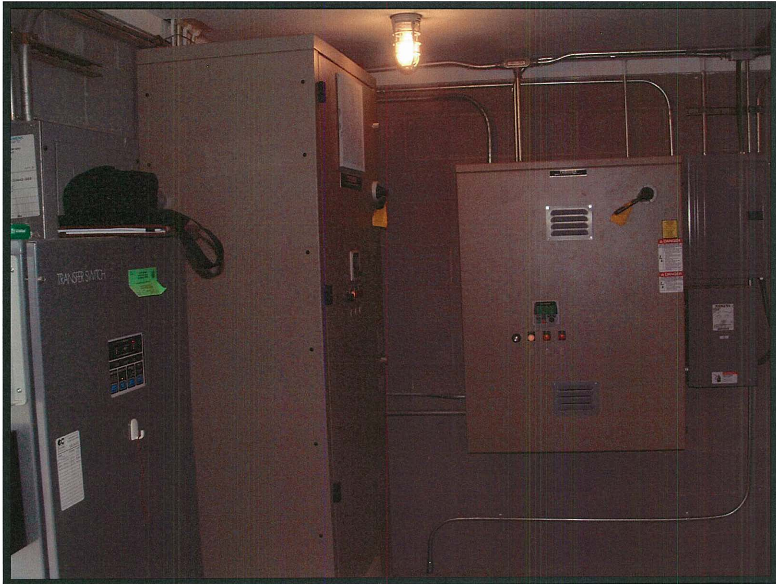
Pump Controlling Works
