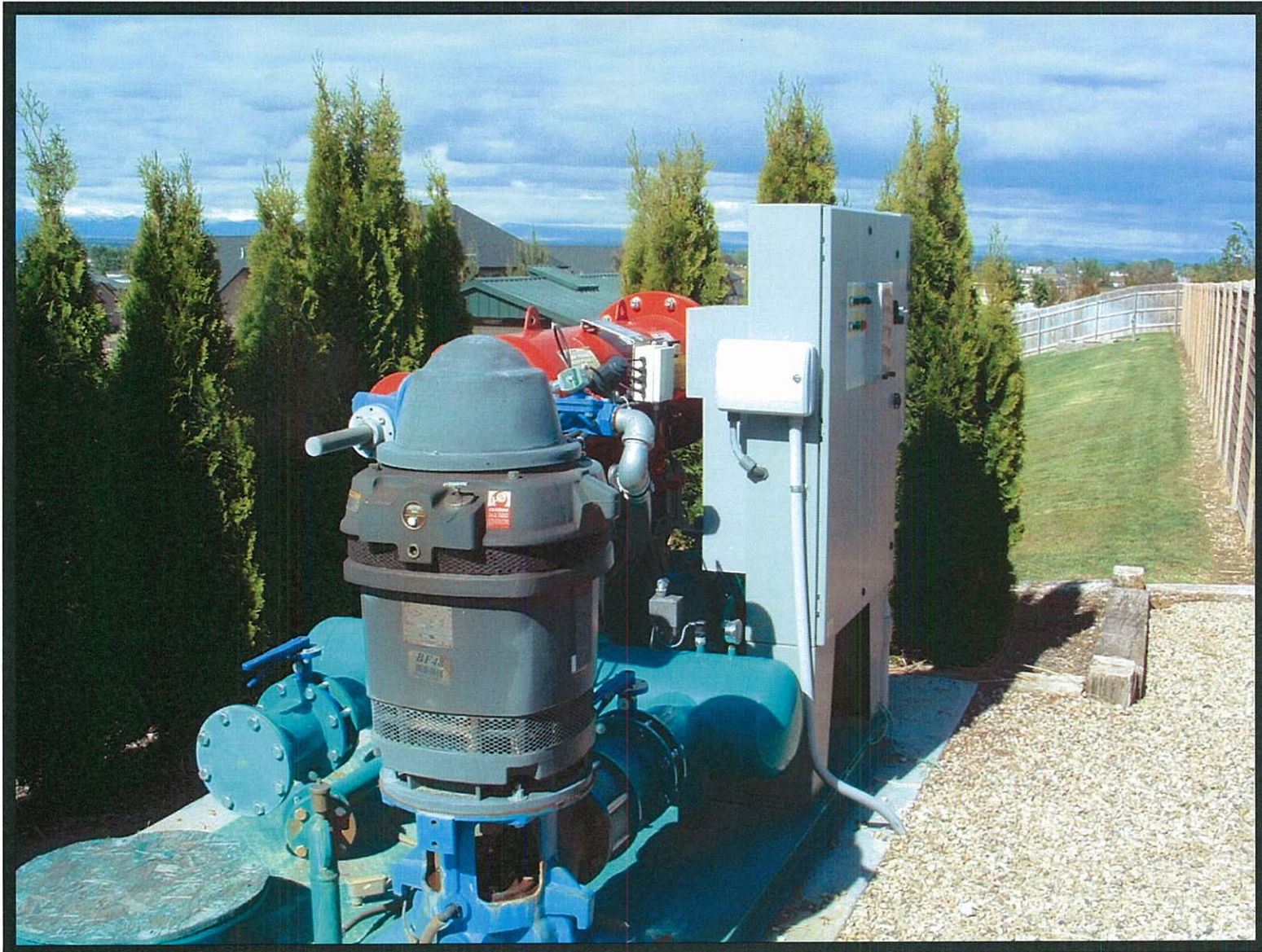
Pressurized Irrigation System
