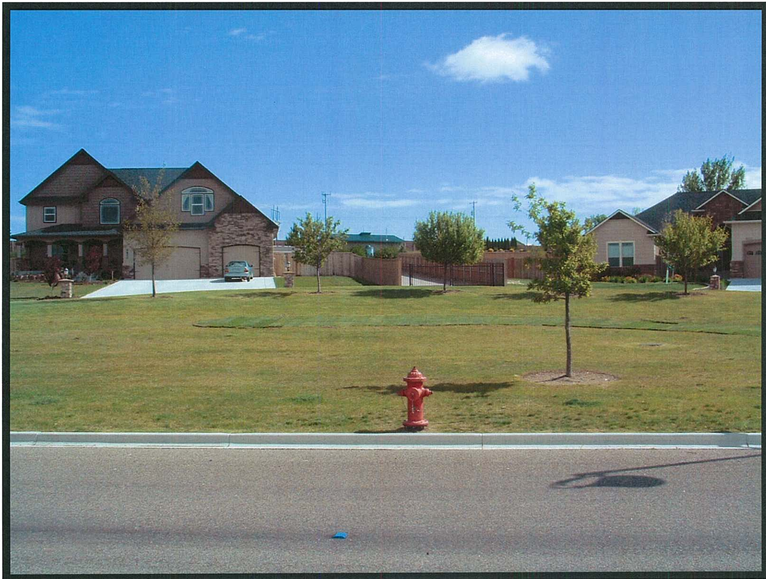
Fire Protection Hydrant
