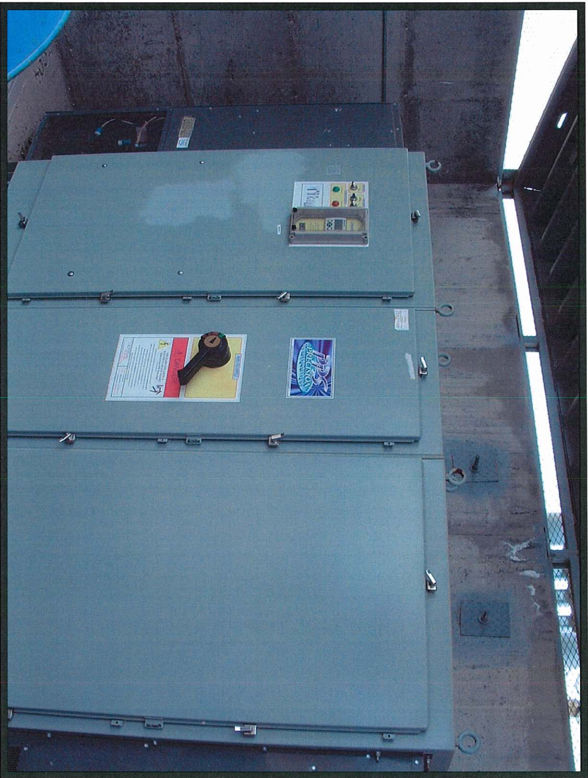
Well 11 Controlling Works
