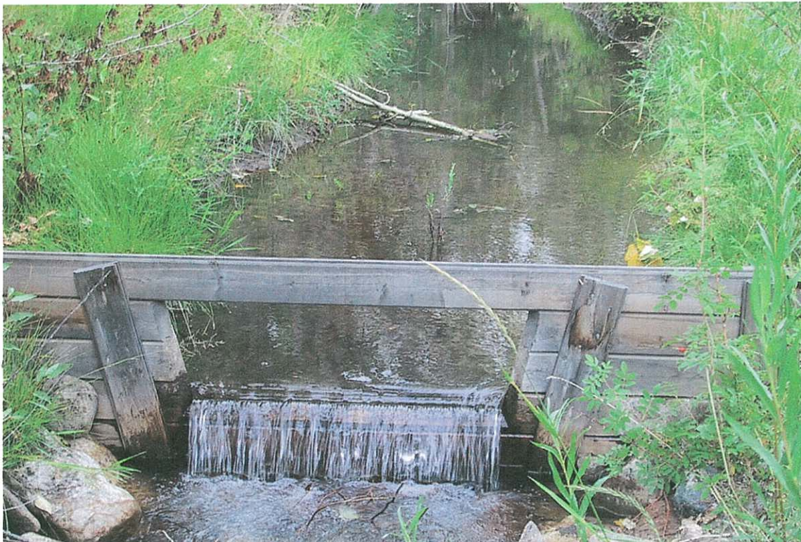
← Cipolletti Weir in Bohannon Creek -6 Ditch
