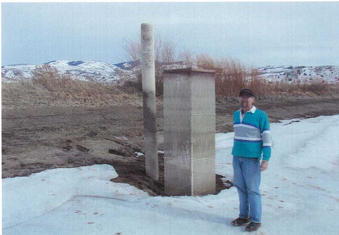
Photo 2 (4/4/08) – Outlet works located in the bottom of the reservoir. In the background is shown a portion of the embankment dam.
