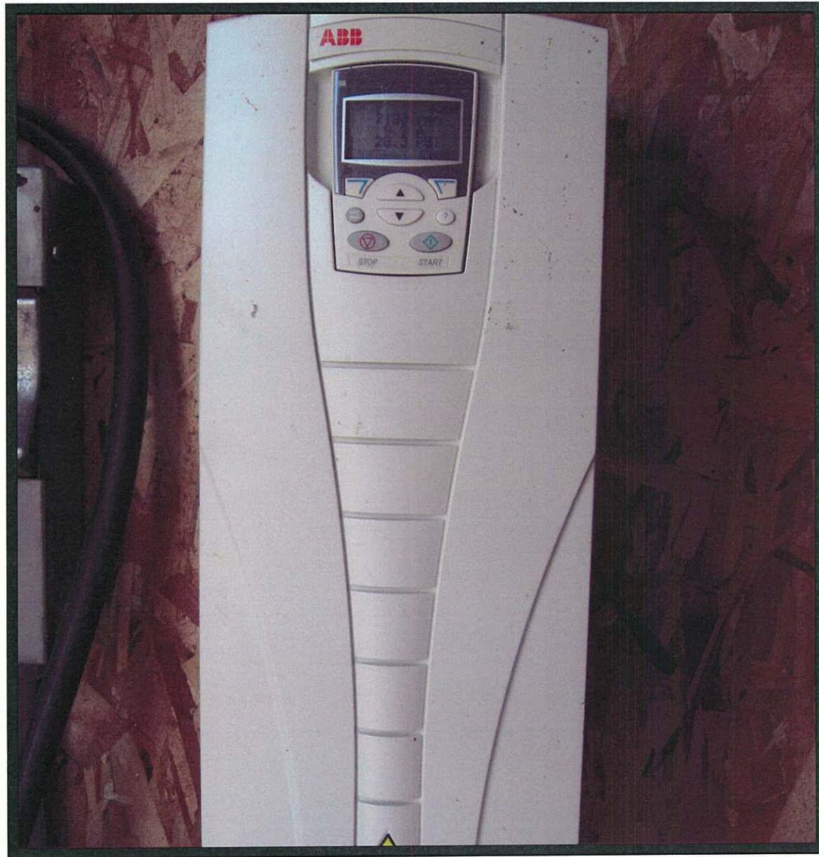
Variable Speed Controls for Well 2
