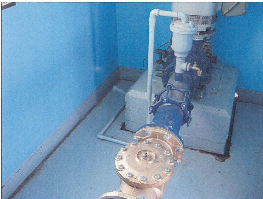
Figure 7: Woodside well pump.
