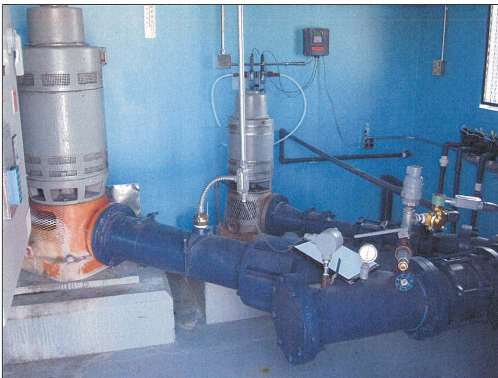
Figure 8: Woodside booster pumps.
