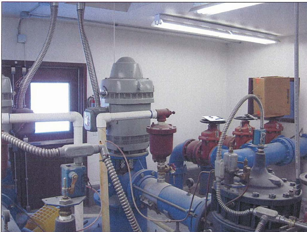
Figure 2: Inside of Northridge pump house with incoming flow from three wells on right and two booster pumps in photo center and left.
