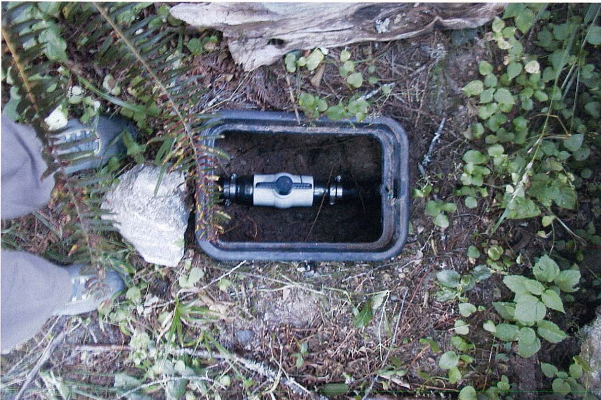
FIGURE 2: Valve control box and 2" PVC pipeline.
