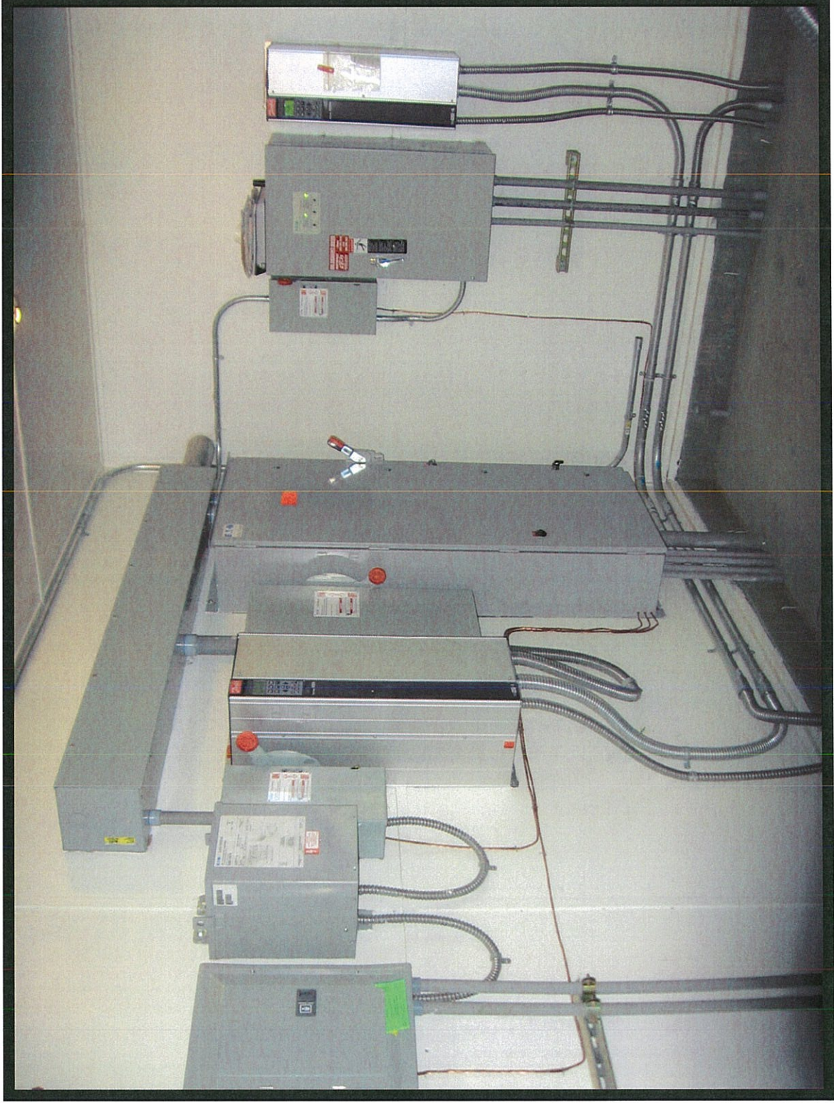
VFD and Main Electrical Controlling Works
