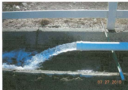
Well discharge entering ditch at 350 gpm from 4-inch PVC
