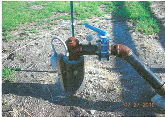
8-inch wellhead in SE corner of property
