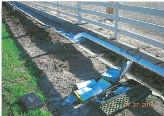
Polysonic flow meter measuring ground water discharge at 350 gpm No surface water in ditch at time of well test
