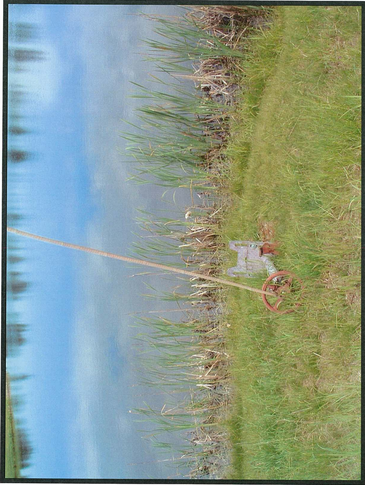
Control Gate for Dam Outlet Pipe
