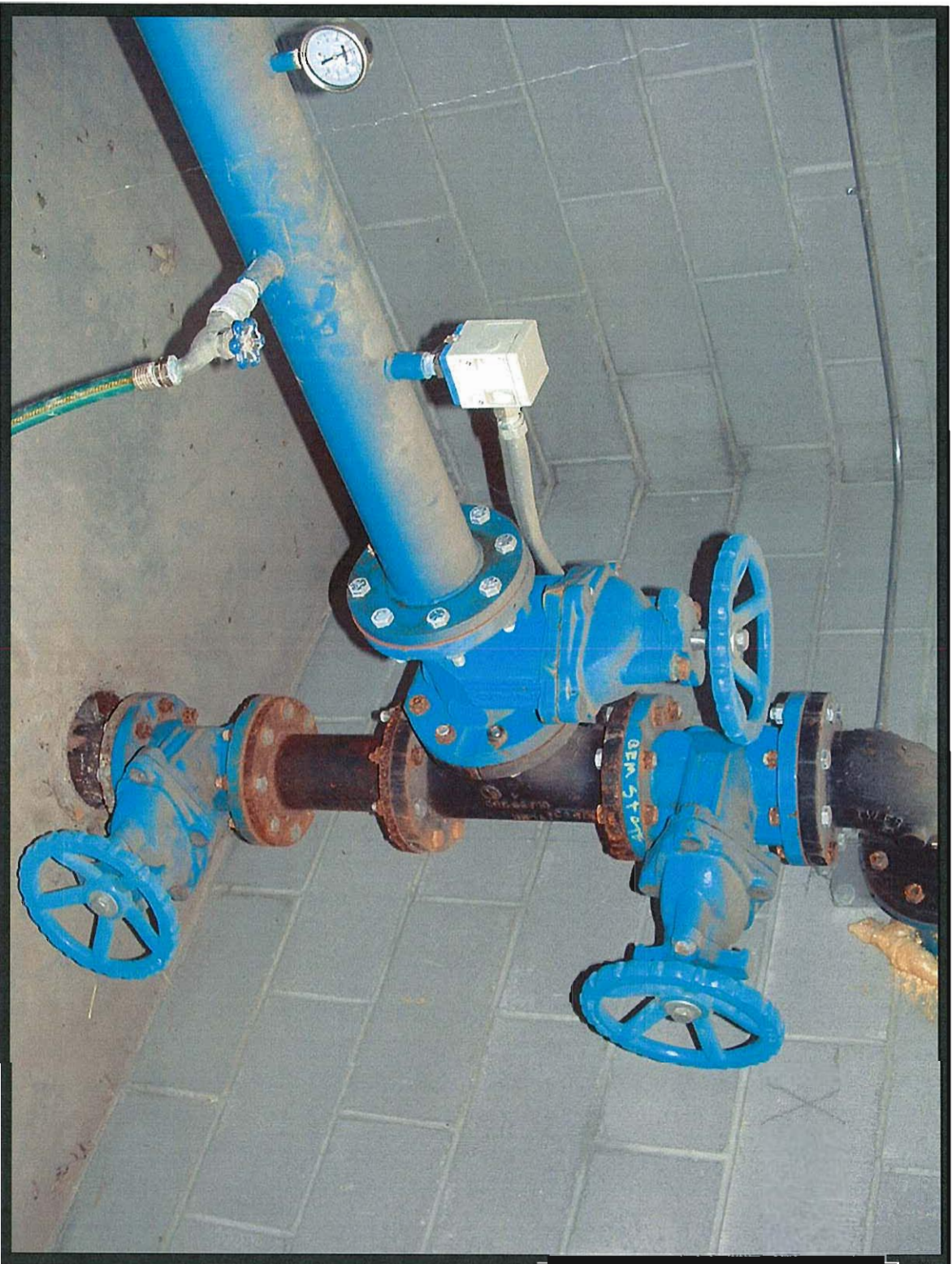
Well 5 Distribution Valves
