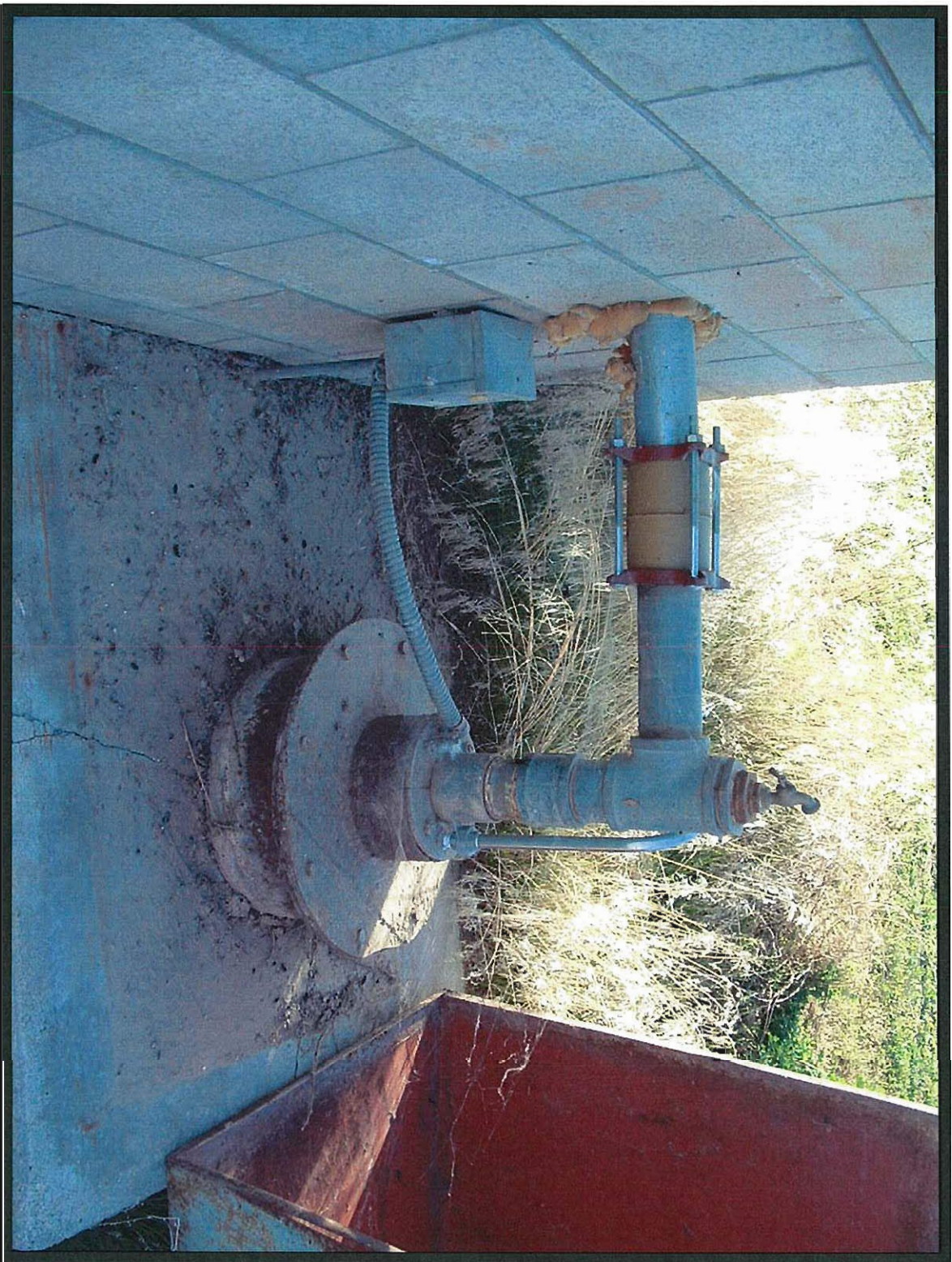
Secondary Well aka Well 1
