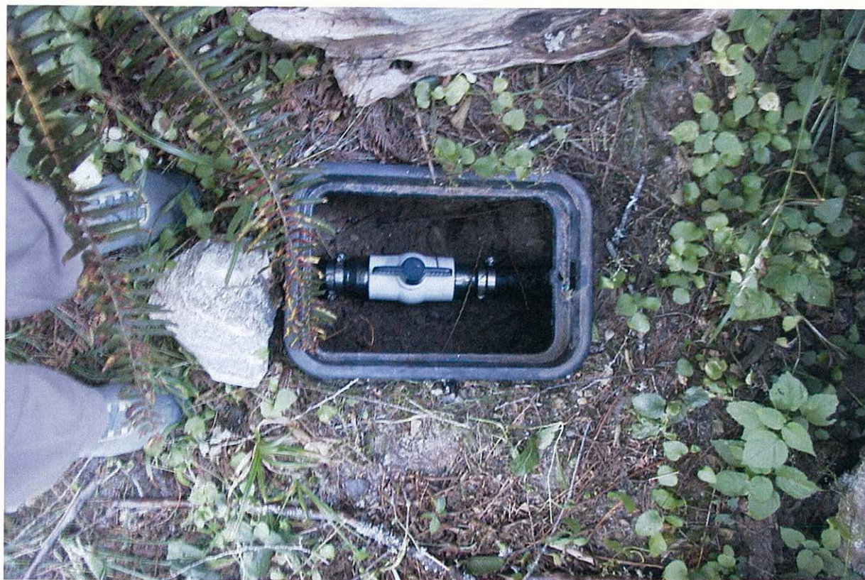
FIGURE 2: Valve control box and 2" PVC pipeline.
