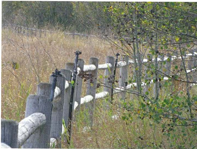
Figure 3. Sprinkler heads located along the fence line on the east side of the property.
