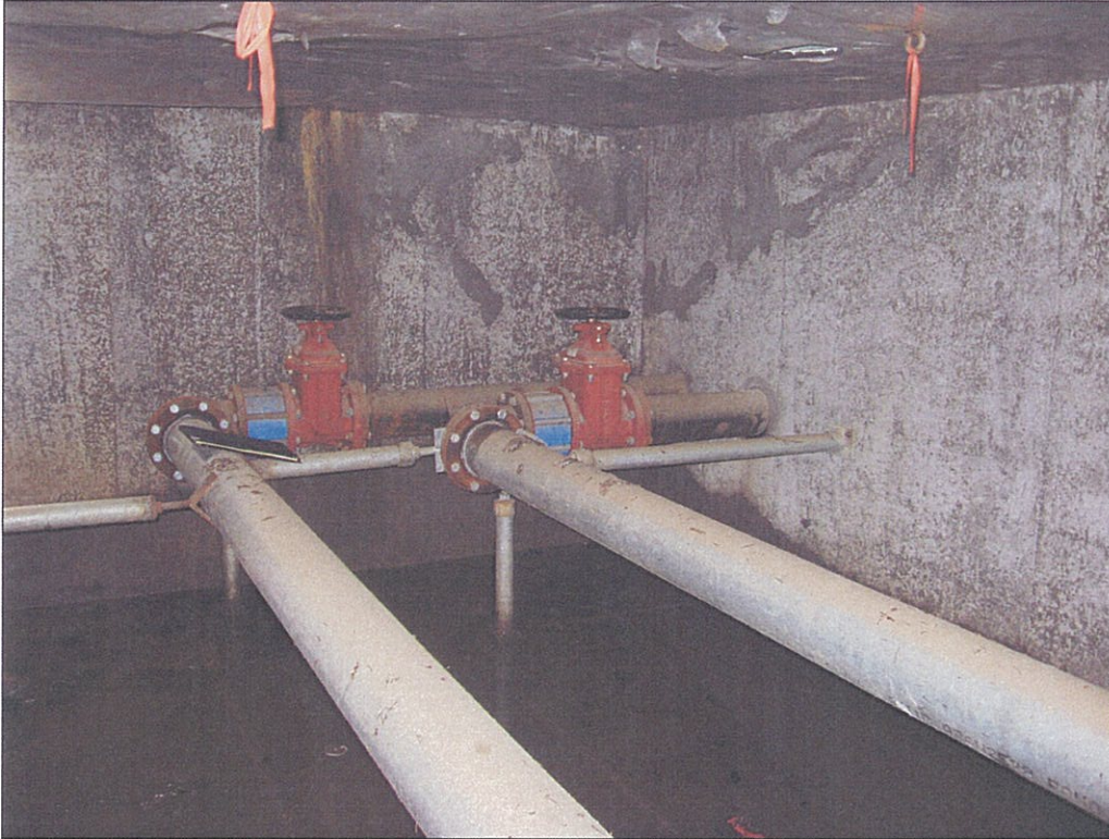
Photo 3: Check and control valves in vault at point of diversion.
