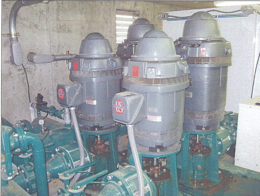
Photo 10: Pumps in the Black Rock Pump Station include two 75-hp (near) and two 100-hp (far) vertical turbines pumping from the irrigation pond.
