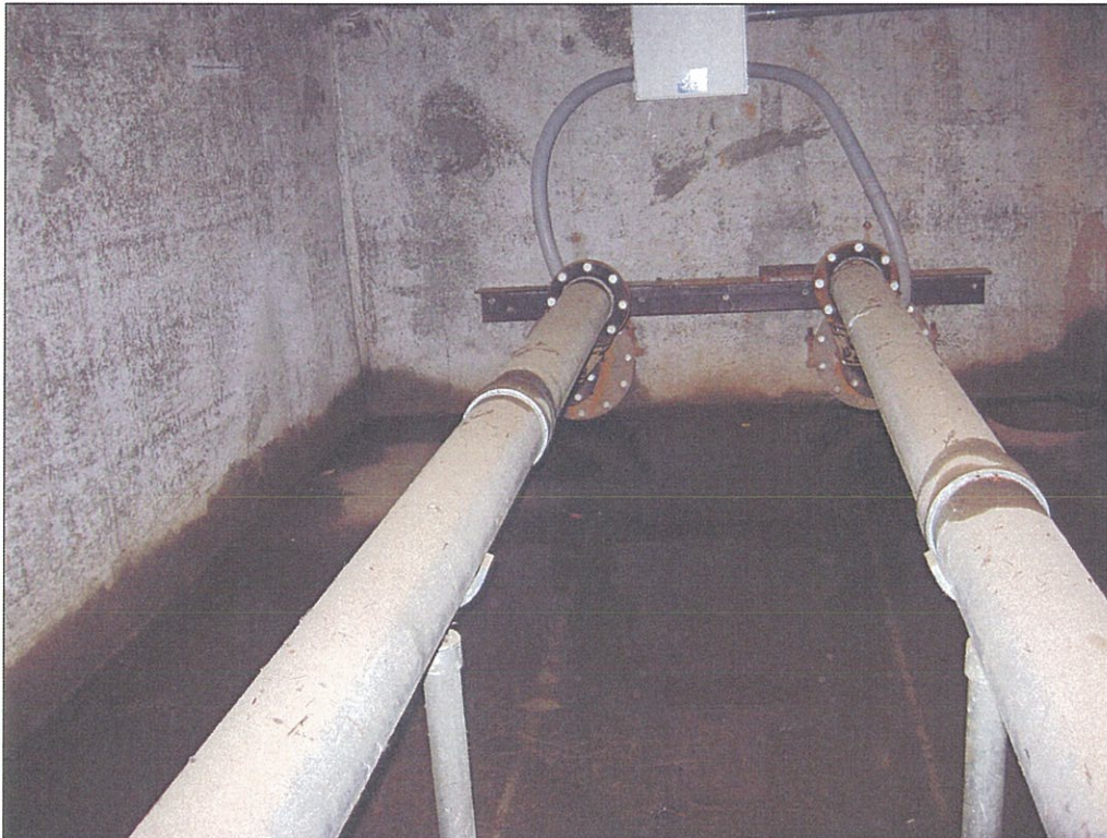
Photo 2: Six inch steel pipelines in vault at point of diversion. Intakes are in the lake.
