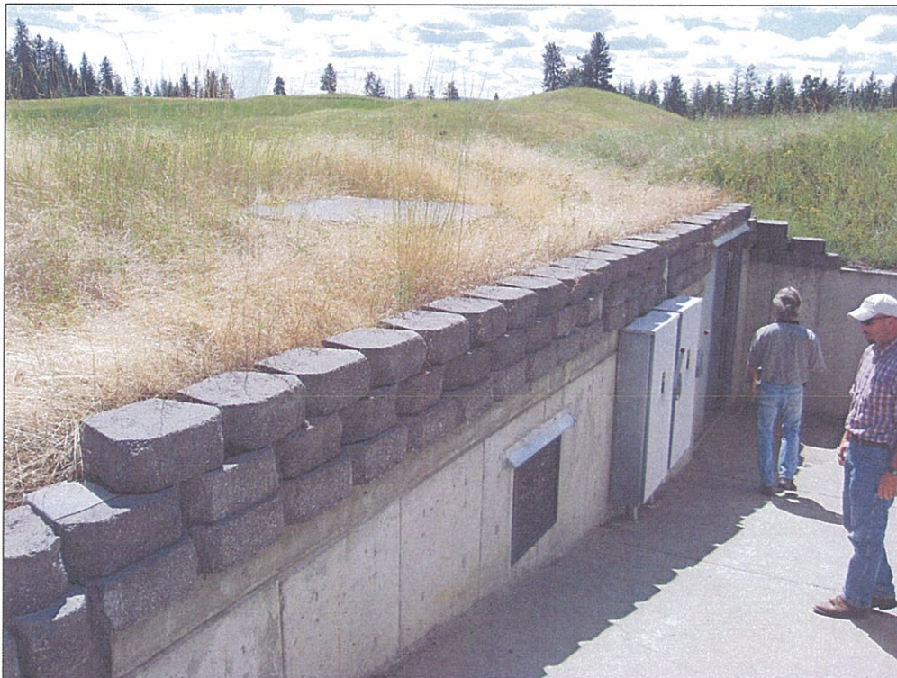
Photo 8: Black Rock Pump Station is located in this vault at the Black Rock Main Irrigation Pond (#9 in the storage features table).
