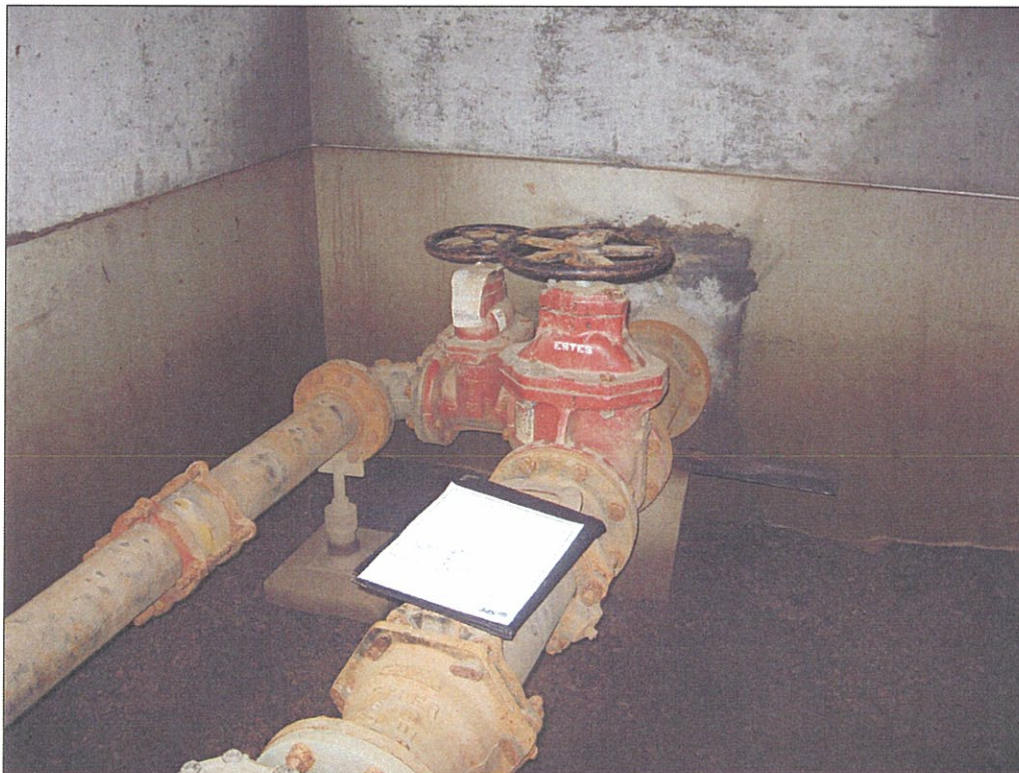
Photo 6: Intake end in the valve and flowmeter vault. The six-inch pipeline on right is primary; the four-inch on left is secondary backup used when flowmeter maintenance is required.
