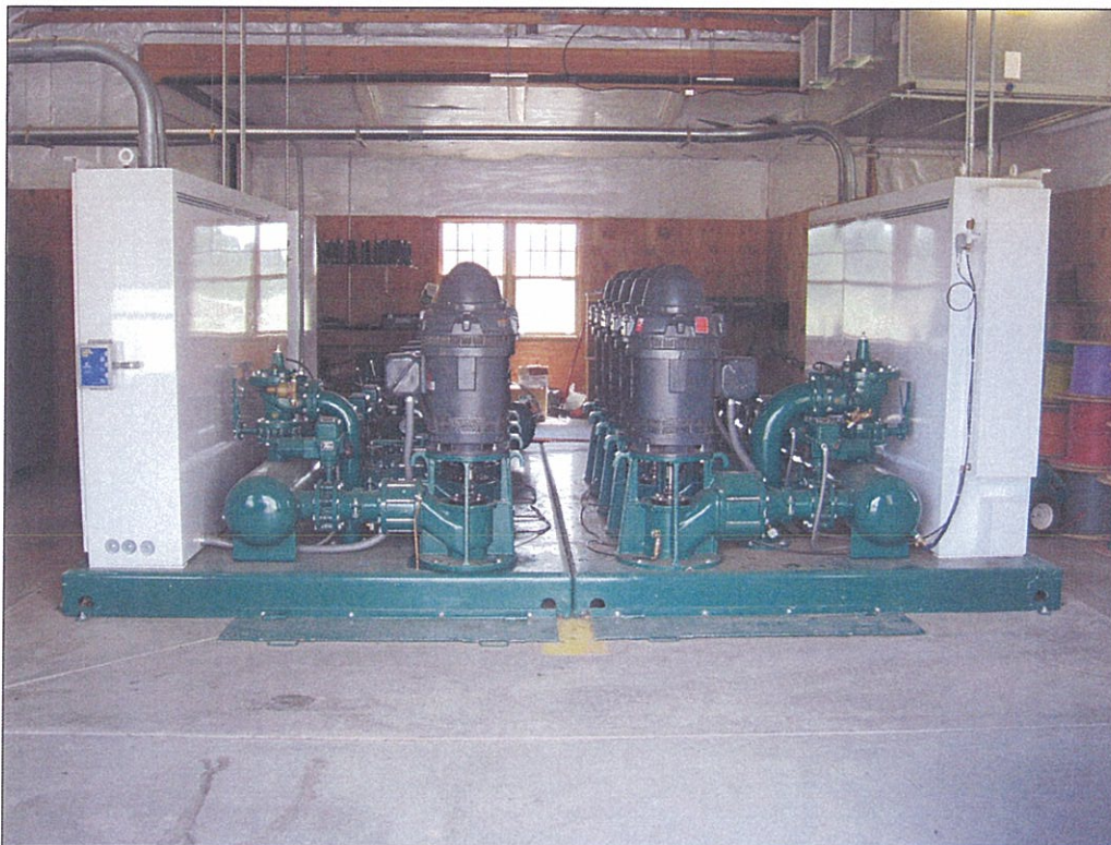
Photo 12: The Black Rock North pump station building is equipped with four 75-hp vertical turbines (left) and five 60-hp vertical turbines (right).
