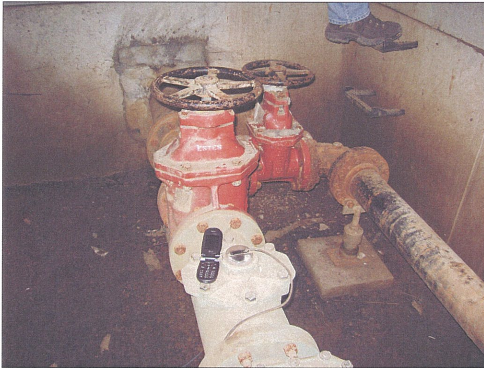
Photo 7: Discharge end in the valve and flowmeter vault. The six-inch Master Meter flowmeter is located upstream of the six-inch gate valve.
