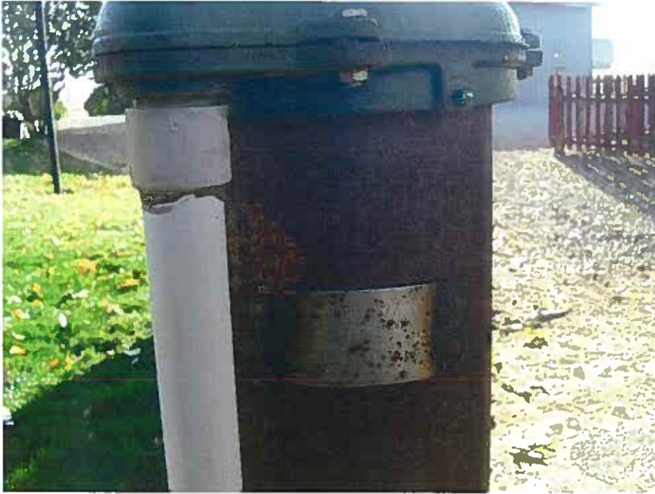
65-23312 License Exam 10/20/2010 Photo #1: Well (POD) with welded Well Tag #D0009432 facing northeast.
