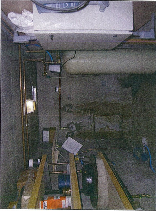
Pic. 9 - Well No. 3 pump house including control panel (right),
