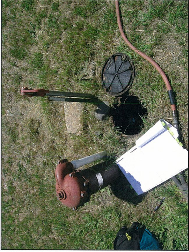
Pic. 2 - Well No. 1 and adjacent totalizing meter vault.
