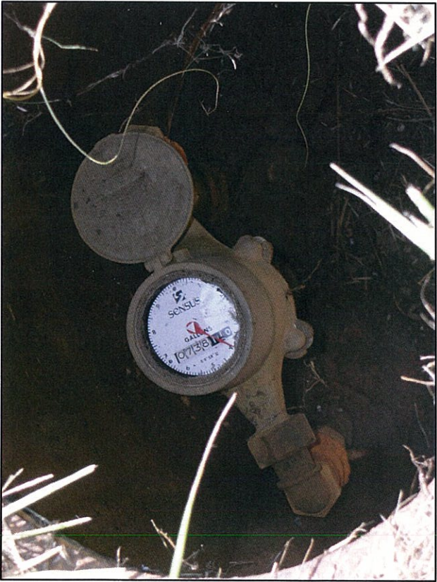
Pic. 1 - Well No. 1 (well ID#284614), Sensus 5/8" SR11 totalizing flow meter (738,120 gallons), services pressure zone 1.
