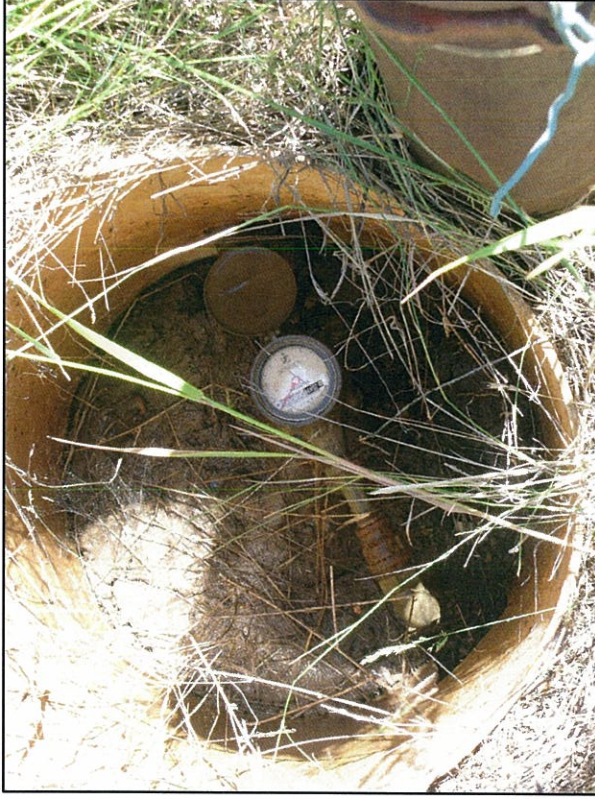
Pic. 6 – Well No. 2 Sensus 5/8" SRII totaling meter (1,594,860 gal.)
