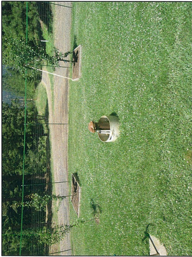
Pic. 11 - Well No. 4 (well ID# 764536) services pressure zone 2.
