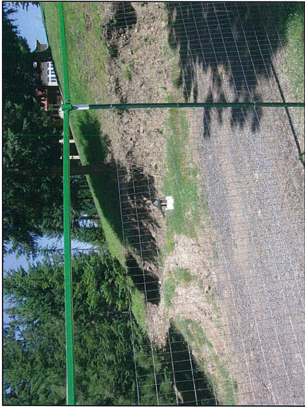
Pic. 12 - Well No. 5 (well ID# 380302) services pressure zone 2.
