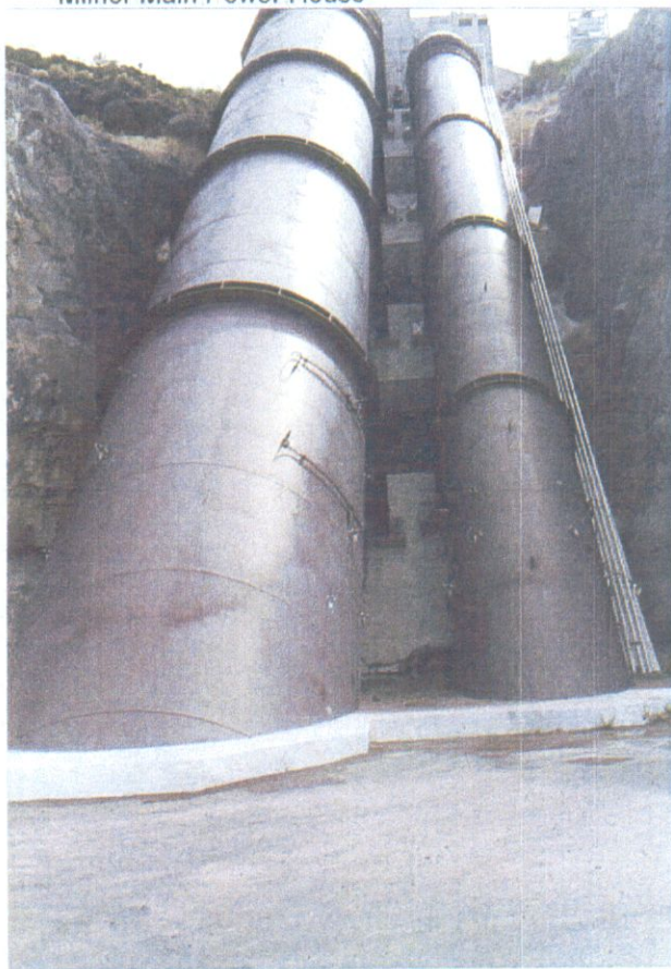
Milner Main Power House Penstocks and Acoustic Flow Meter Taps
