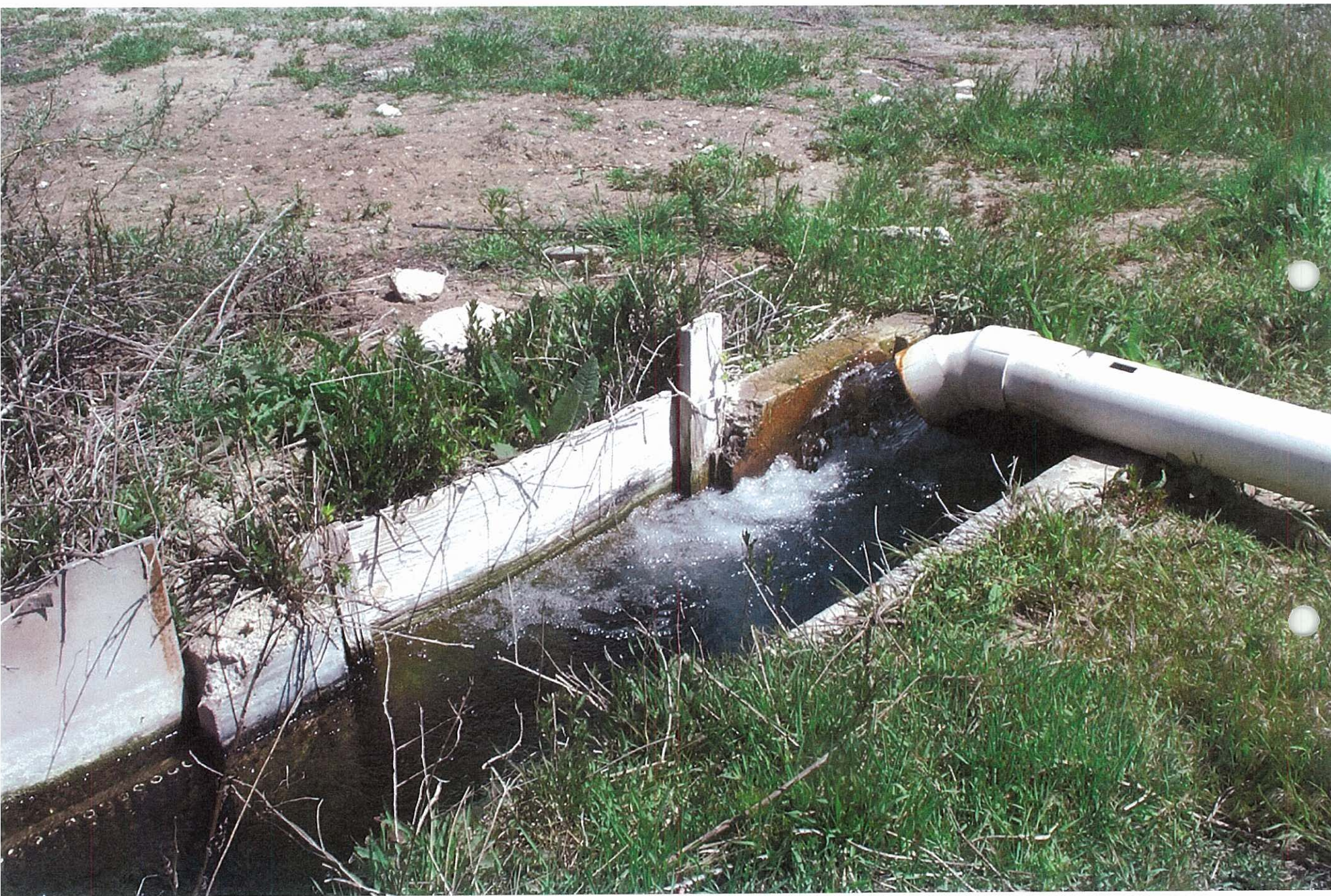
47-7659 Pipeline From Upper Raceways To Inlet For Middle Raceway 5-19-08 By J Stanton Looking N
