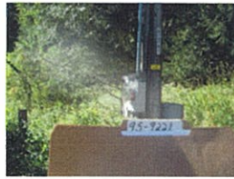
pump controler and power meter.JPG
