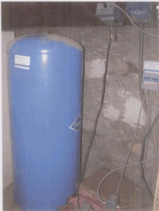
Figure 2: Pressure tank for well system.
