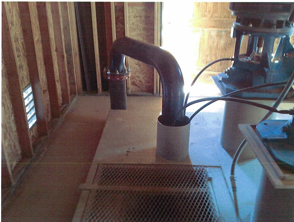
Photo 2: Inside well house showing discharge pipe leading from well to wet well (center); one of the re-lift pumps is shown at right
