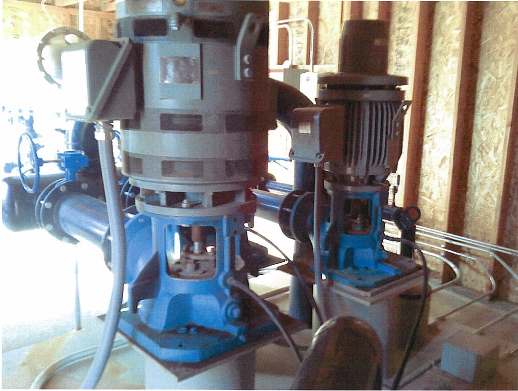
Photo 3: Re-lift pumping system; discharge pipe from well is in foreground
