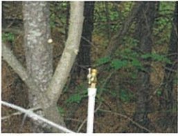
water line to POU.JPG
