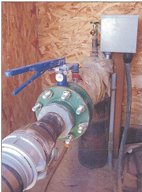
Photo 2: Eight-inch well, pressure transducer for variable speed drive control, four-inch discharge piping, 4-inch butterfly valve, and connection to flexible delivery hose.
