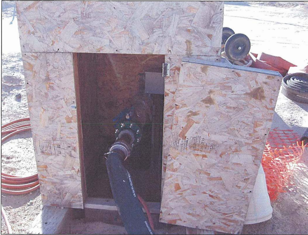
Photo 3: Well, pump house, and discharge piping.
