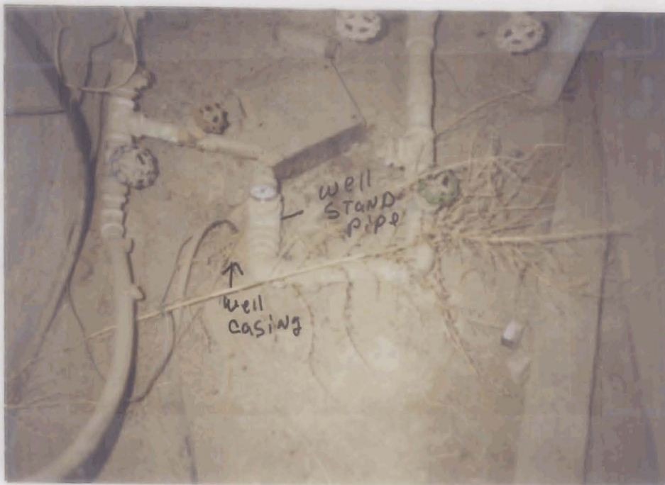
This is the well for well #2. The casing is covered with dirt.
