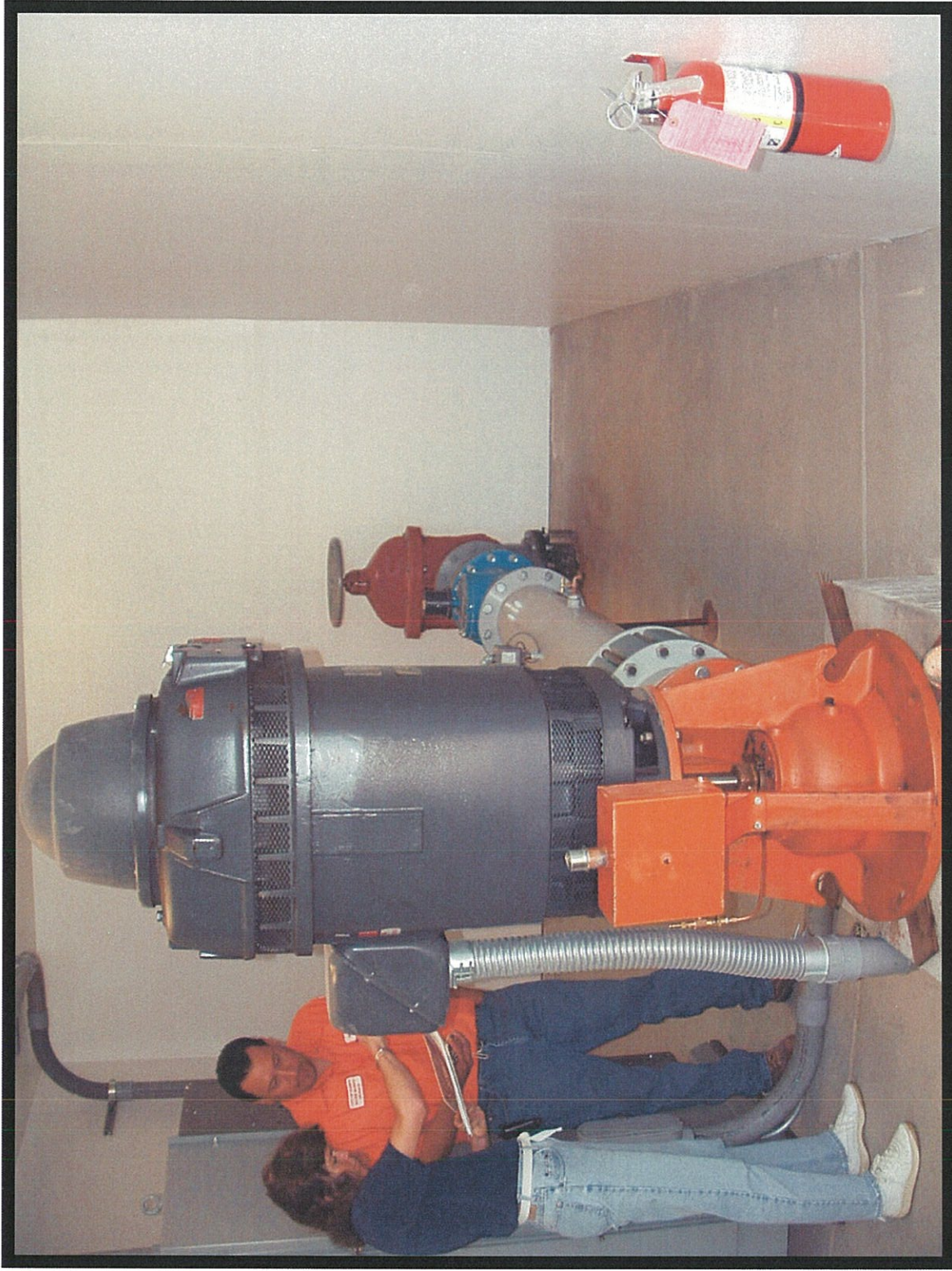
16-inch Well and 200 HP Turbine Pump
