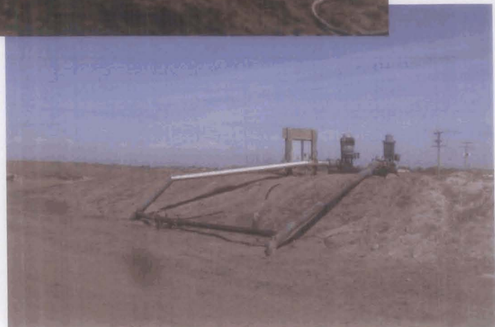
view of relift array with supply pipelines heading north and south
