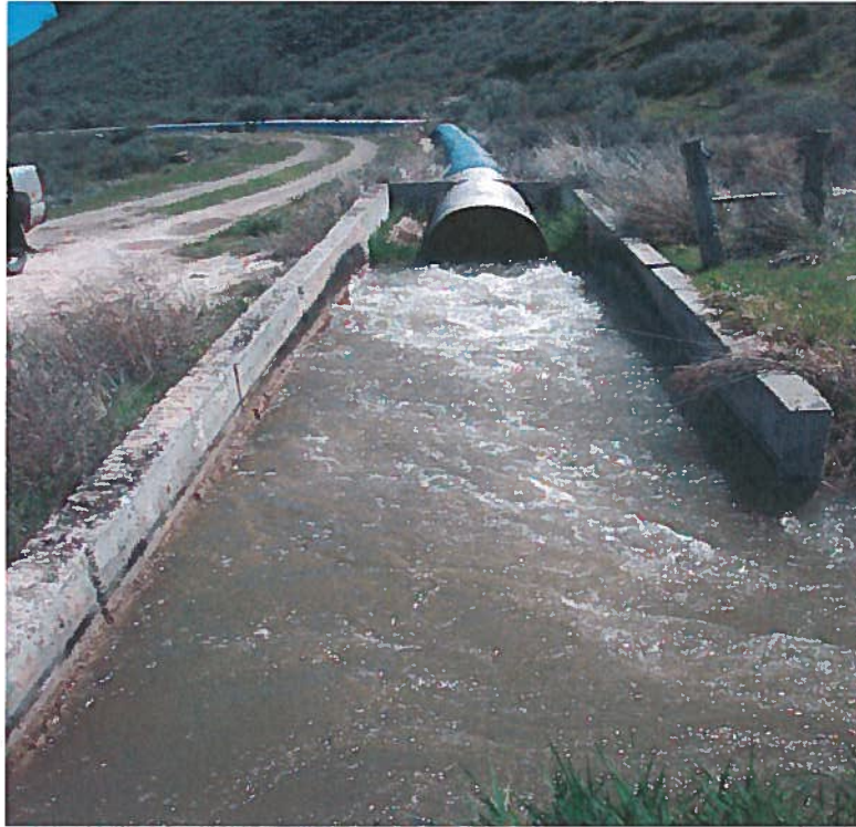
Figure 3: Discharge into facility
