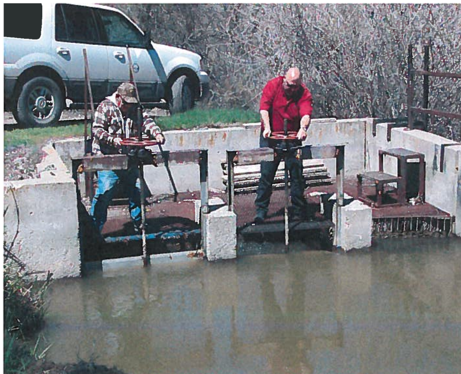
Figure 2: Opening head gates at point of diversion
