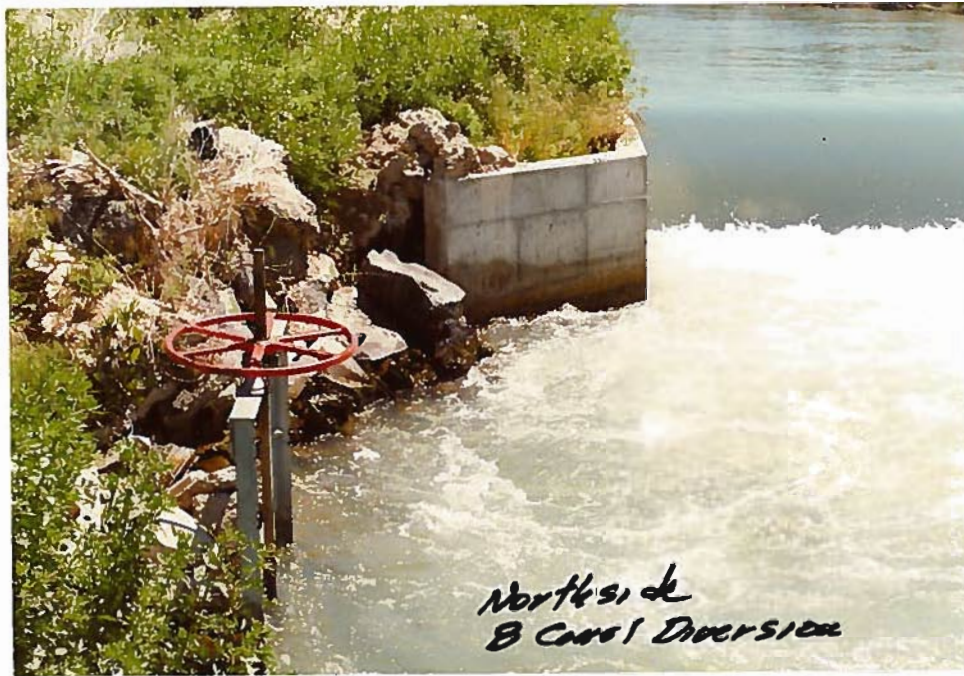
B Canal Diversion - Headgate
