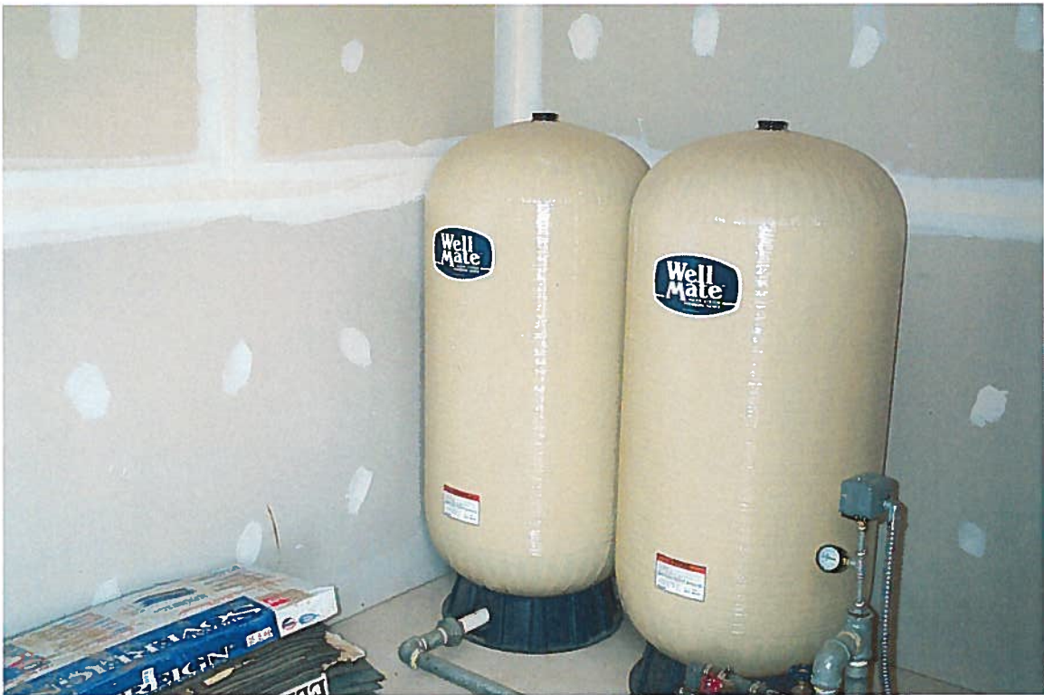
Pressure Tanks Behind Well By J E Stanton 3-18-05
