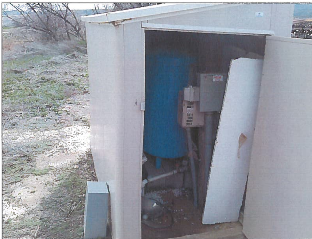
Figure 4: Well #2 inside pump house.
