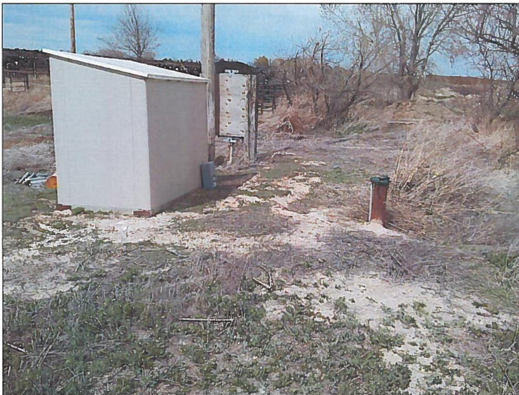
Figure 3: Well #2 and pump house (on left).
