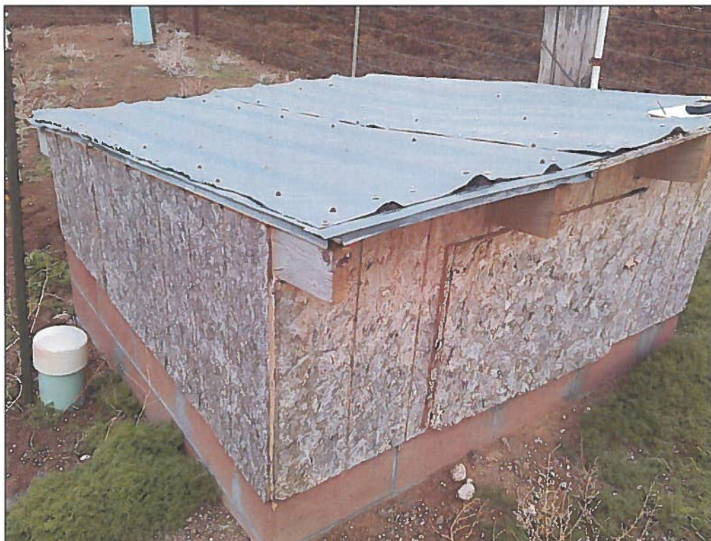
Figure 2: Well #1 pump house.
