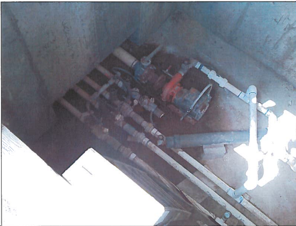
Figure 14: Pump and control for 10,000-gallon storage facility.
