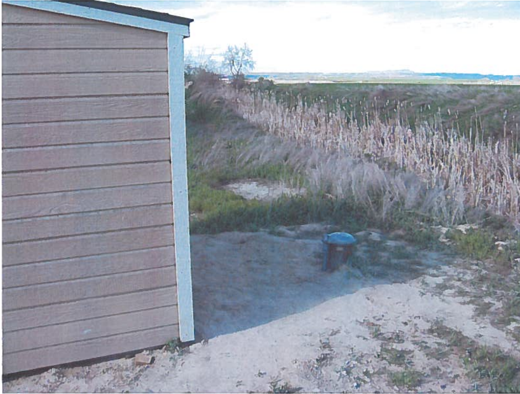
Figure 5: Well #3 and pump house.
