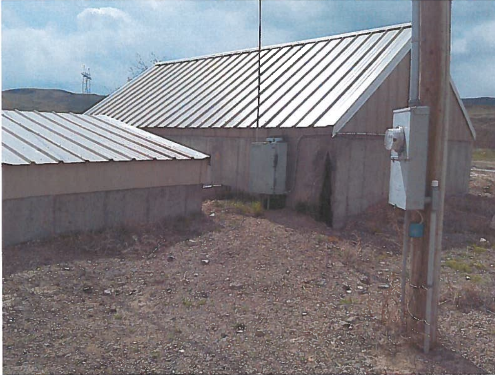
Figure 13: 10,000-gallon storage facility.
