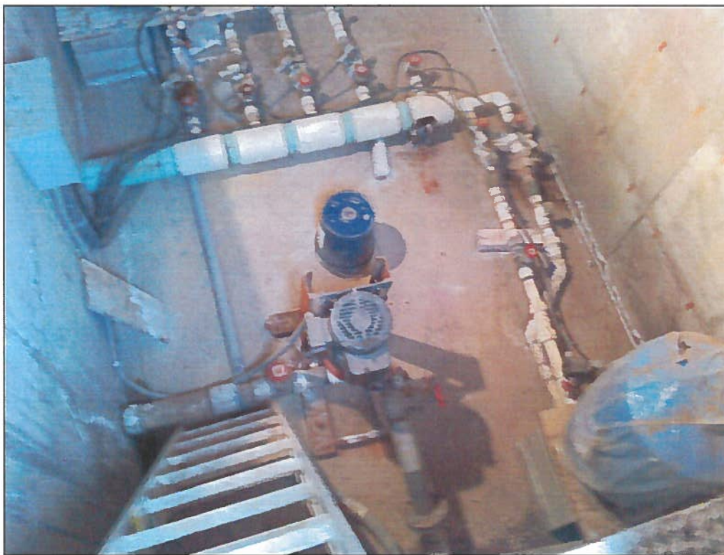
Figure 8: Pump and controls for 50,000-gallon storage facility.
