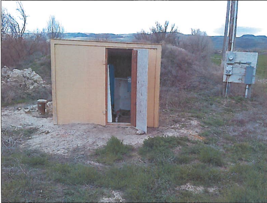
Figure 9: Well #5 and pump house.
