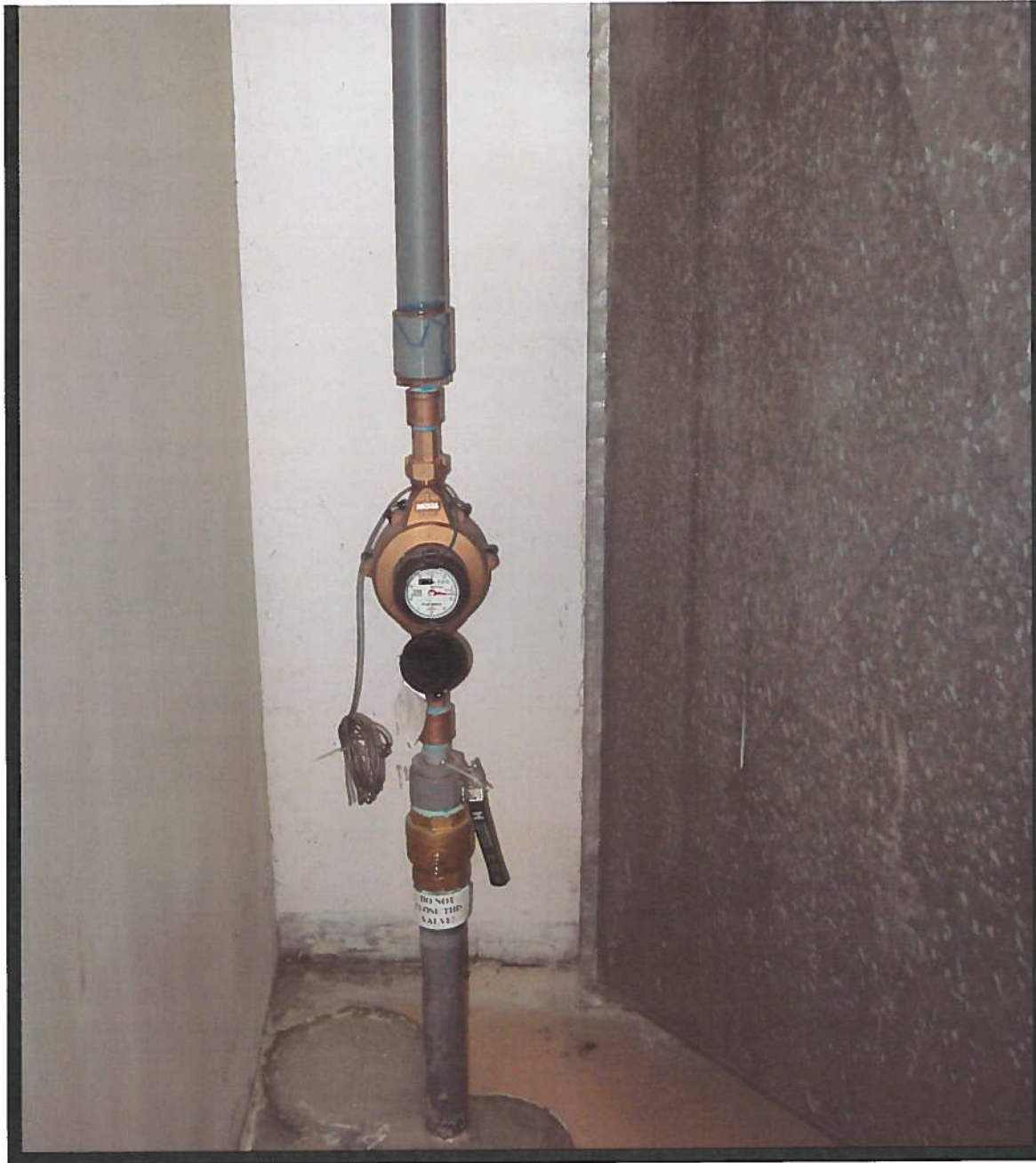
Ground Water Supply Line and Flowmeter
