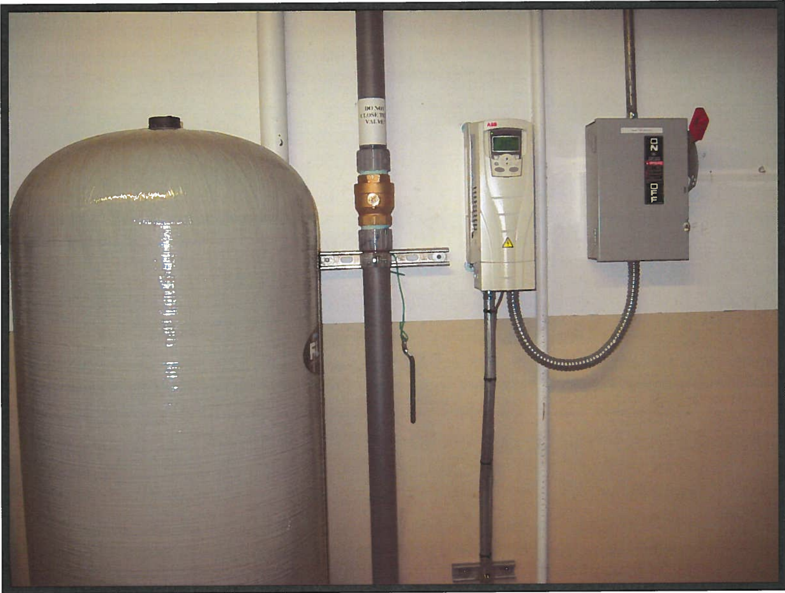
Submersible Variable Speed Pump System Controls
