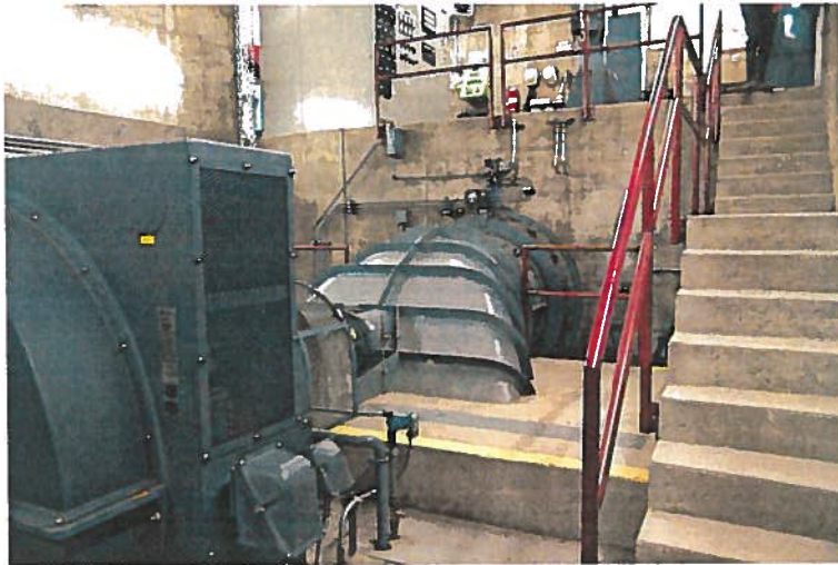
View of Generator in foreground with exposed portion of turbine in background with control equipment on deck above. Photo taken looking upstream from within power plant.
