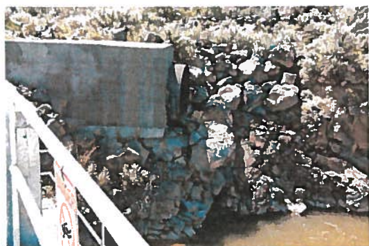
Emergency bypass pipe used whenever plant goes offline. This is reported to be a newer feature at facility to prevent interruption of flows in Little Wood River.
