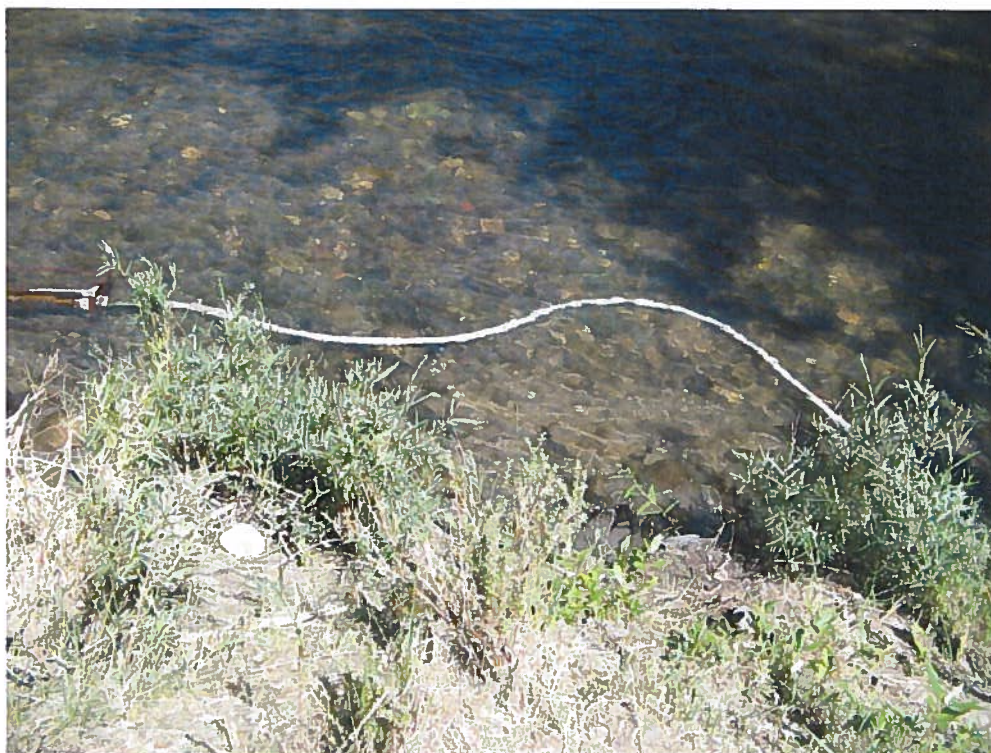
This is the actual intake from the river. The river is flowing from right to left. The intake is shown at the left. A required fish screen is in place. 1.5-inch pipe goes from the intake to the pump and then is throughout the system.
