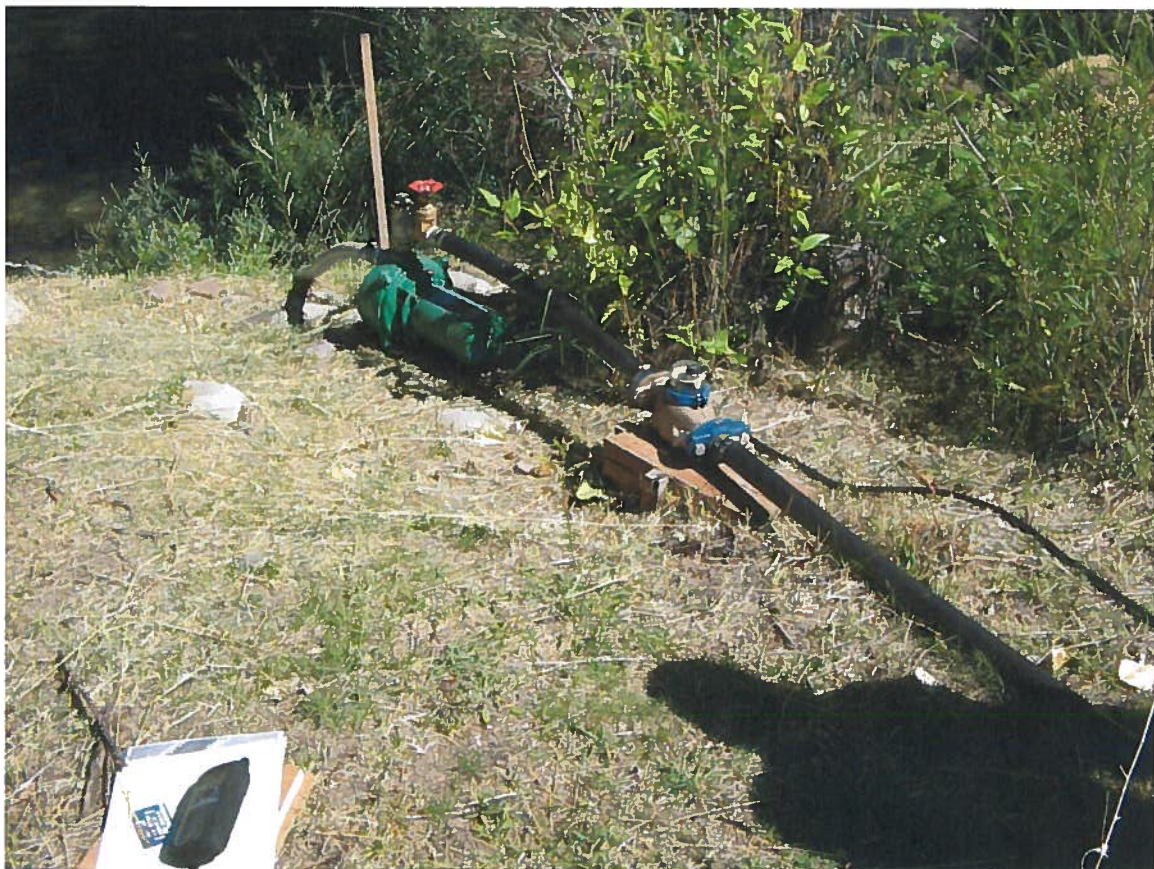
A0017301 (2502202 1519499). Point of diversion. Picture taken looking southwest. The river is available in the background. Pump is a Myers with a 1.5hp GE motor. There is an installed meter shown with a blue arrow. The installation of a measuring device is a condition of the permit, and Mr. Oldham sends regular meter readings.
