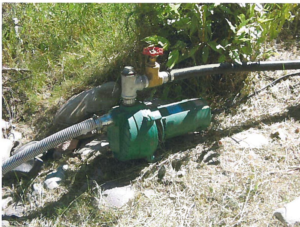
Close-up of the pump apparatus.
