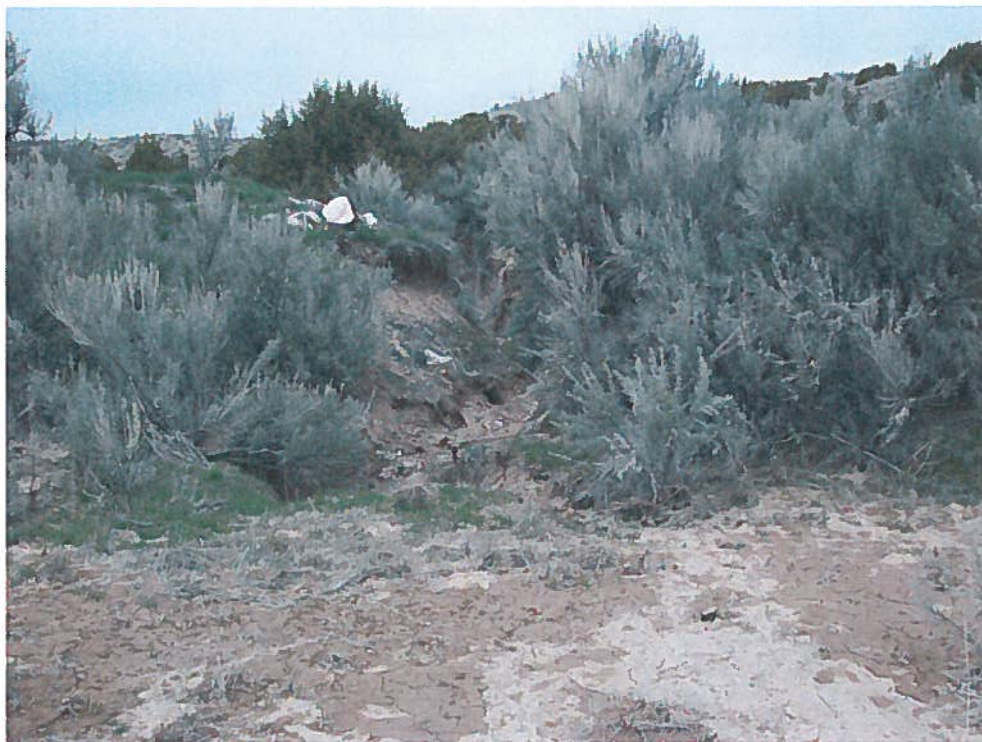
Figure 5: Eroded Spillway on lower reservoir
