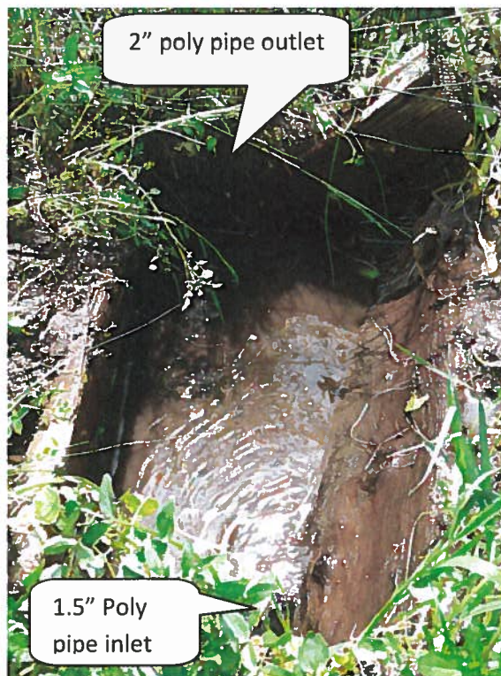
Figure 2: Headbox after removal of vegetation.
