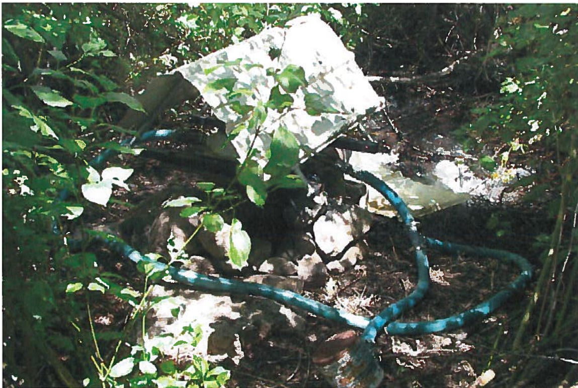
Hydroelectric generator, inlet hoses, and relation to Lower Rock Creek.
