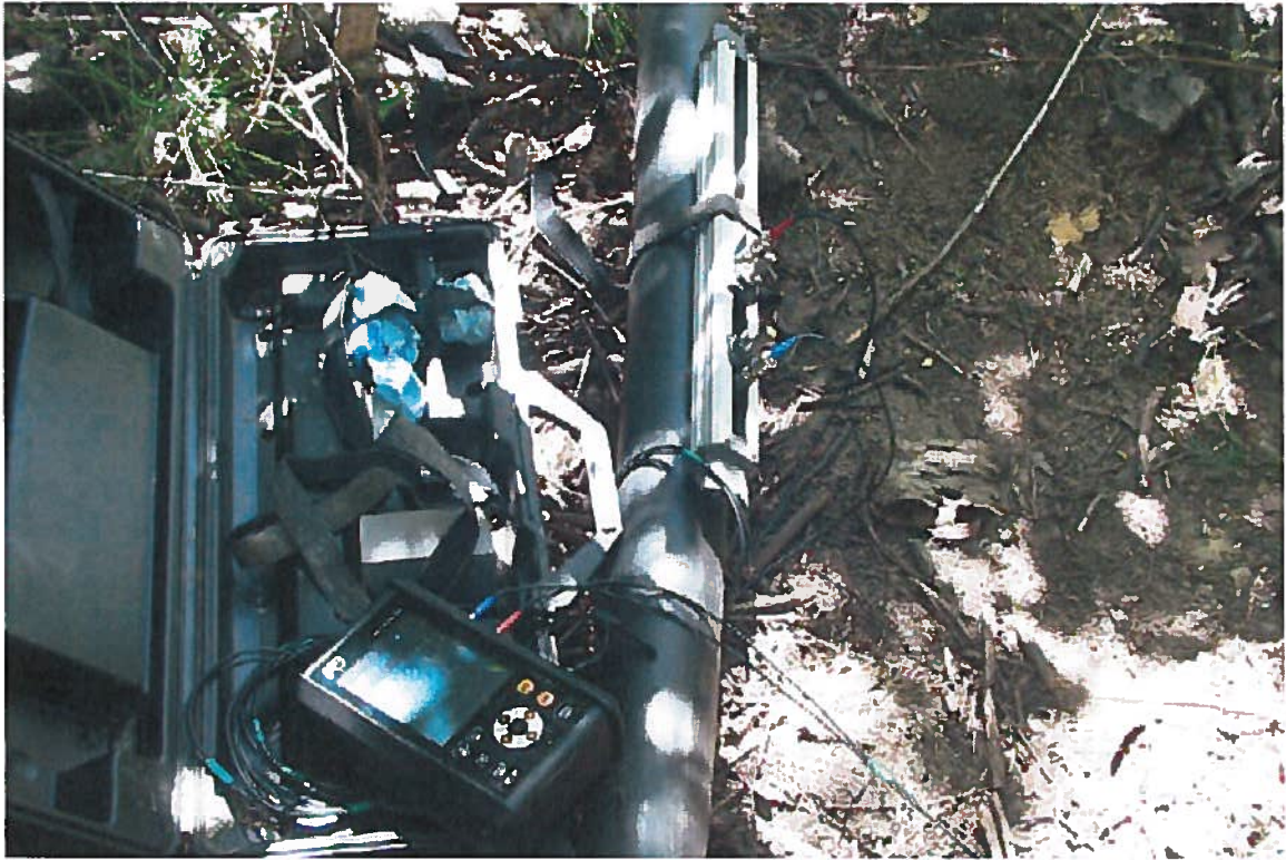
IDWR Flowmeter attached to pipe above generator.
