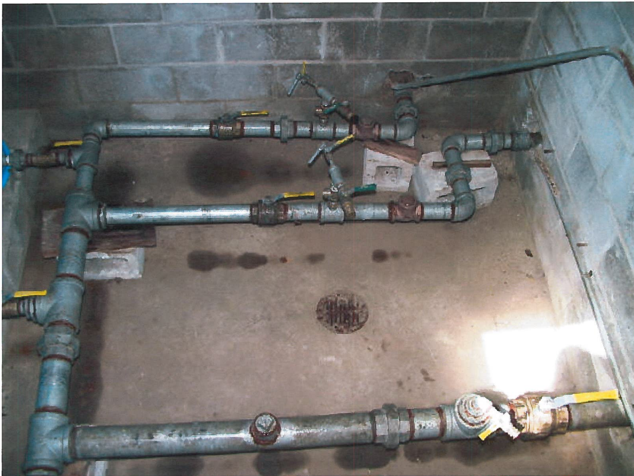
Snake Traps Plumbing in 10x11 House
