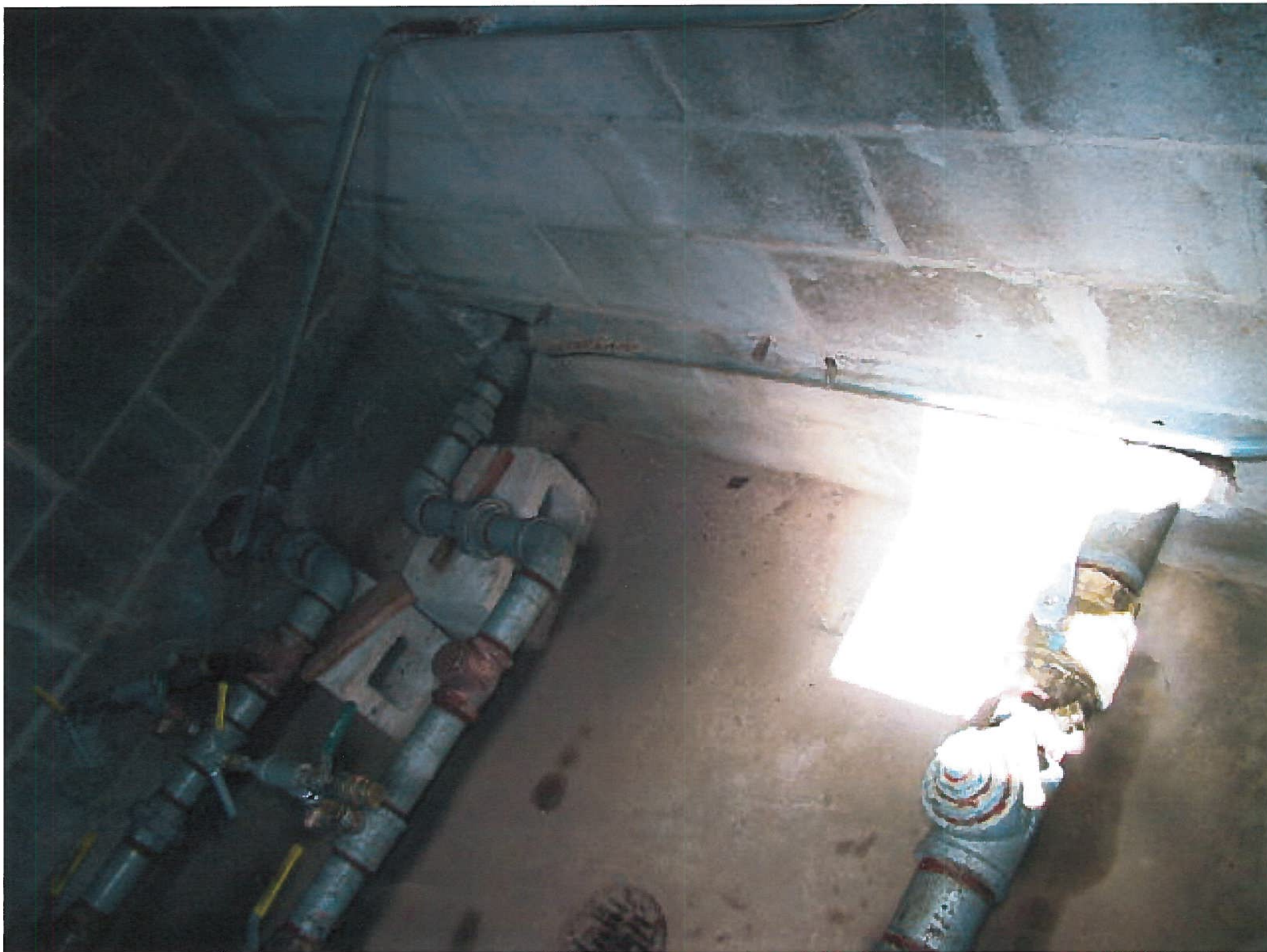
Space Acres Plumbing in Well House
