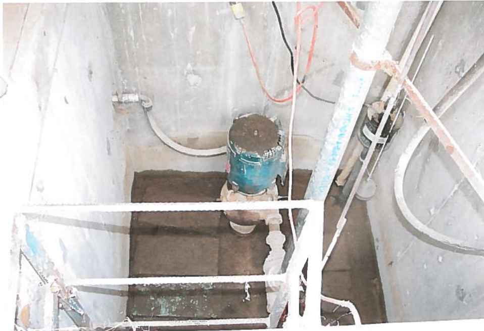
Pump for diverting water to the orchard
