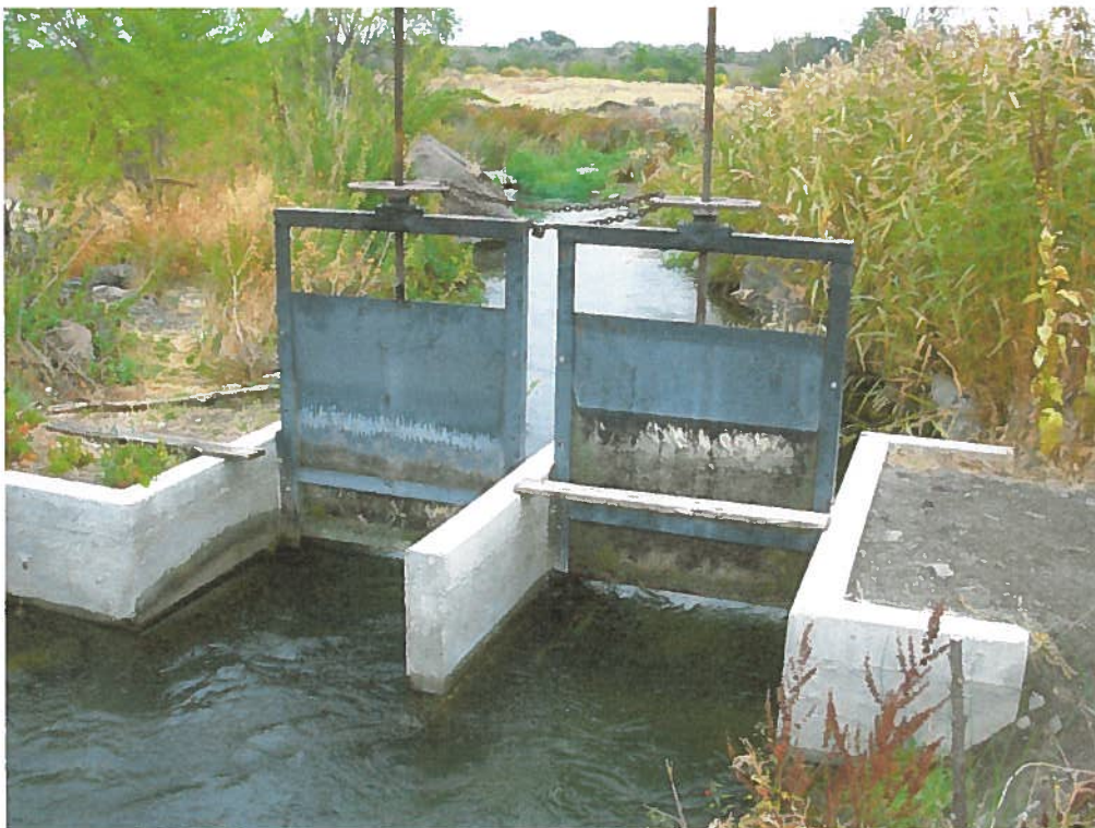
Lockable Slide Gates at Hunt Ditch Head – Looking Upstream
