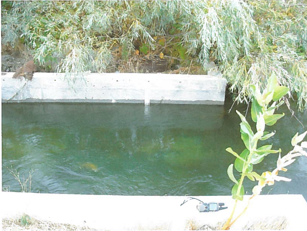
Staff Gage on Weir Wall – Stilling Well Behind Staff Gage
