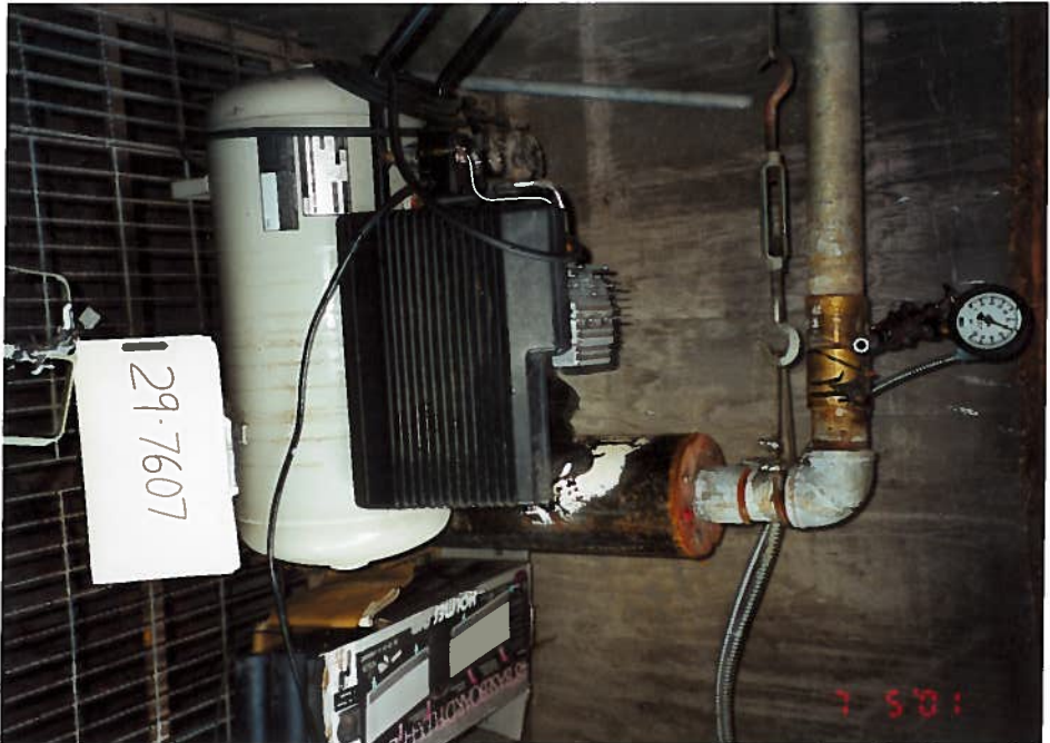
Well #1 inside well house
