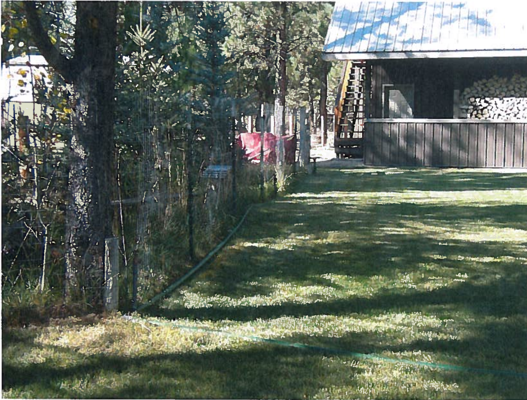
Permit holder's place of use – note sprinkler lines are not buried
