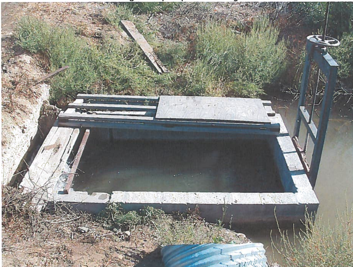
Headgate and weir box for Upper Haas Ditch. Baldridge and Meadows Drain to the right, Upper Haas Ditch to the left.
