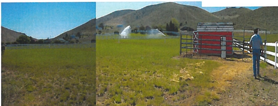
Well and pump house. Irrigation to left and right of pump house. Well is white tube sticking out of ground with a 15hp sub. 35hp in house.
