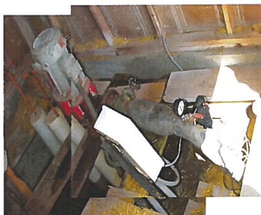
35hp booster pump.
