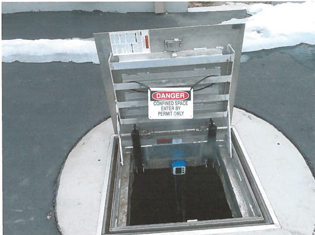
Figure A2: Hatch to vat room meter. Similar configuration for Well 4.
