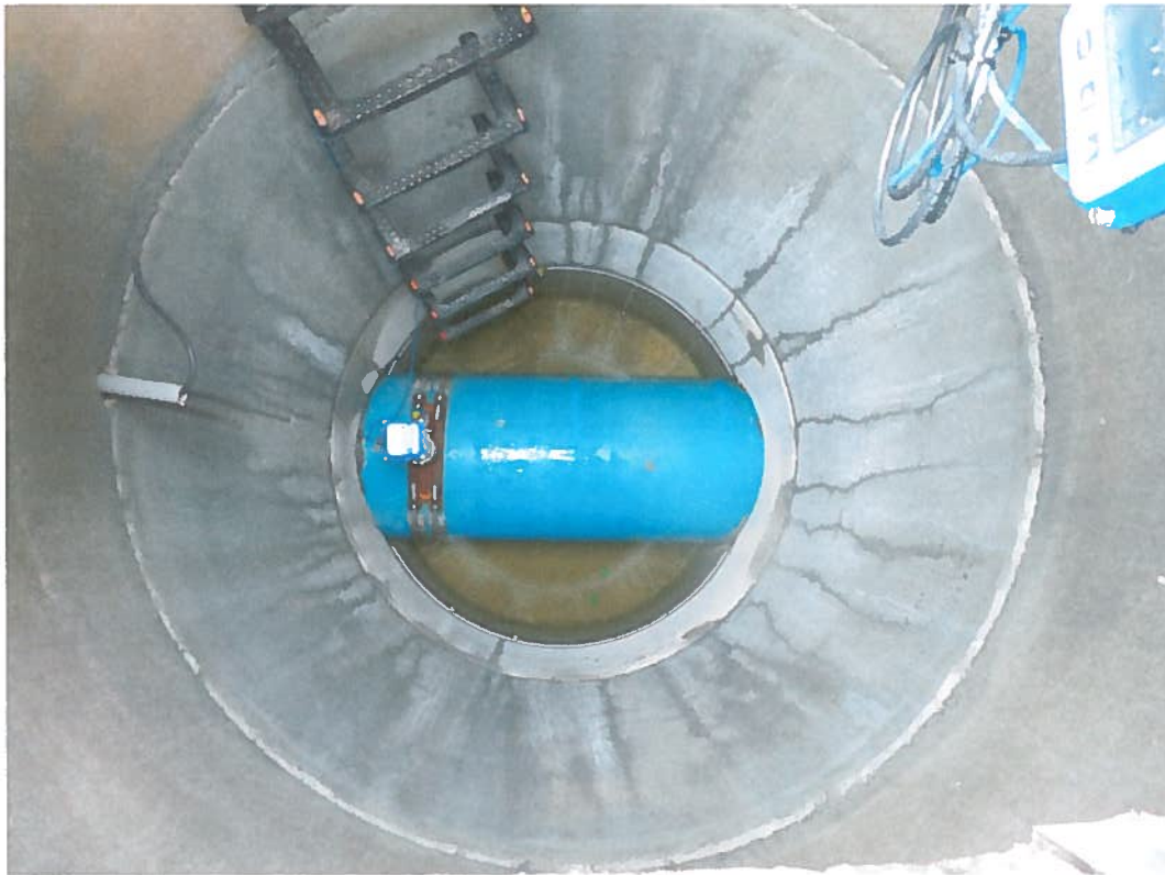
Figure A4: SeaMetrics meter on line to VAT room.
