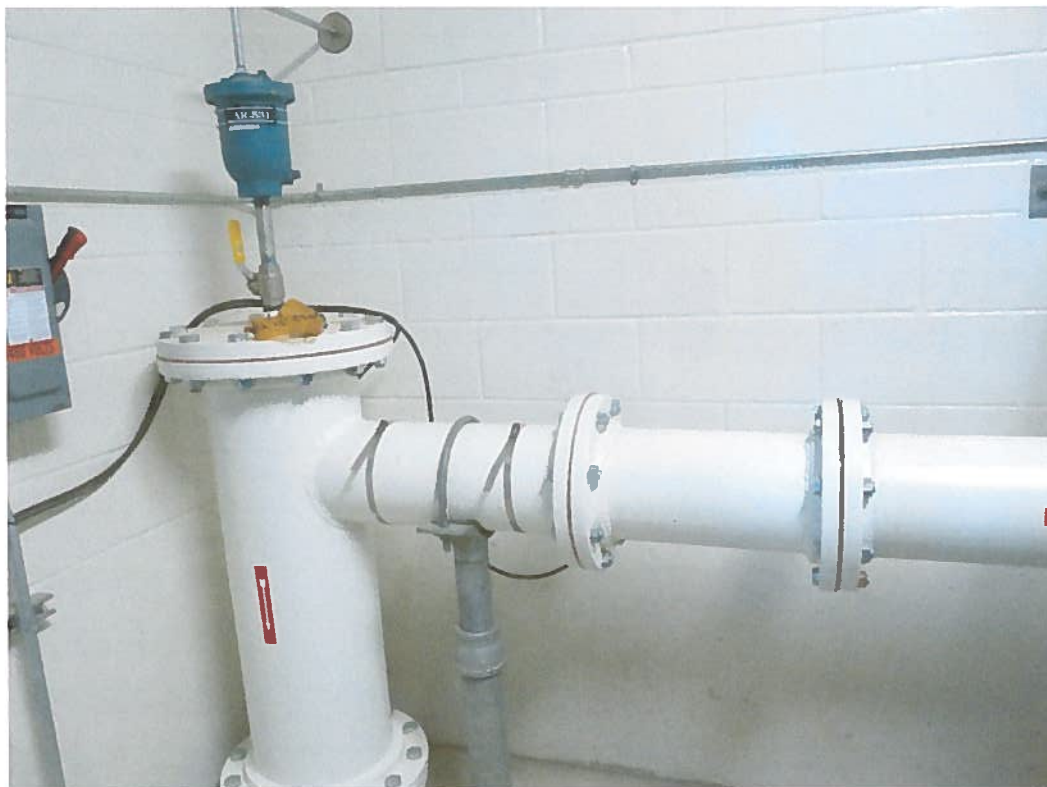
Figure A1: Meter placement on Well 3. This configuration is similar to that of Well 2.
