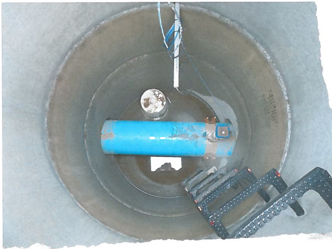
Figure A3: SeaMetrics meter on Well 4.
