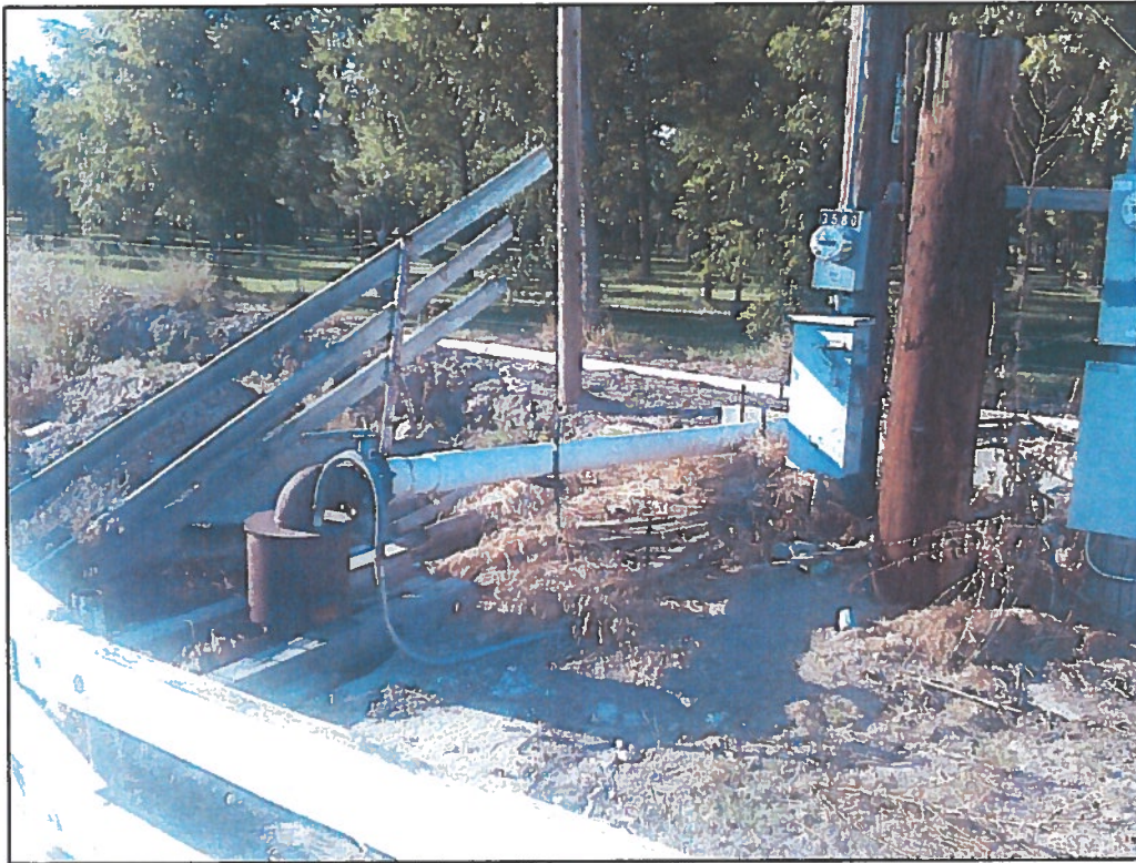
Well, in lower left of photo, is equipped with a submersible pump discharging through a six-inch PVC pipe into the McMullen Lateral.
