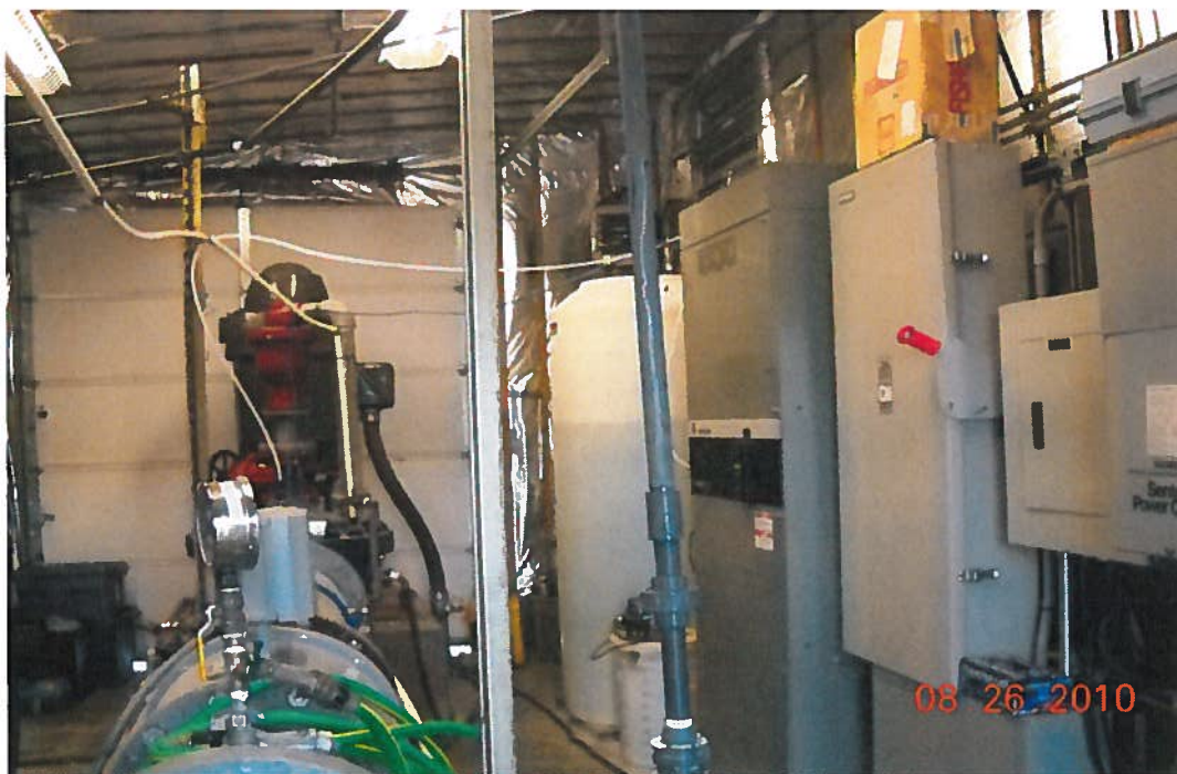
Inside wellhouse. Well is at far end of building.
