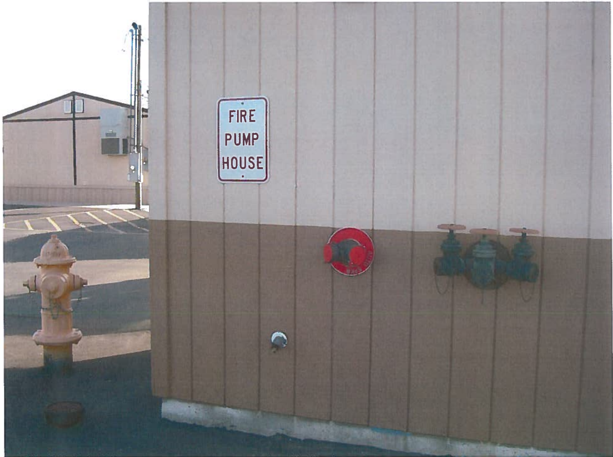
63-31131 License Exam 10/22/2010 Photo #3: Fire hydrant and hose hookups outside fire pump house, where well is, facing northeast. One of several school buildings in the background (main building to the east/northeast of fire pump house).
