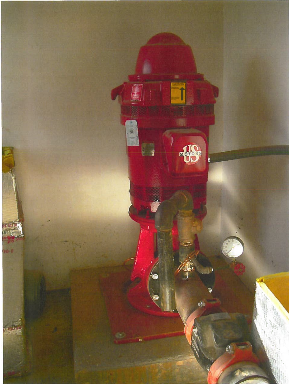
63-31131 License Exam 10/22/2010 Photo #1: US Electric motor (Serial # H060S2BLG) mounted on well head. Note pressure gage with release pipe.
