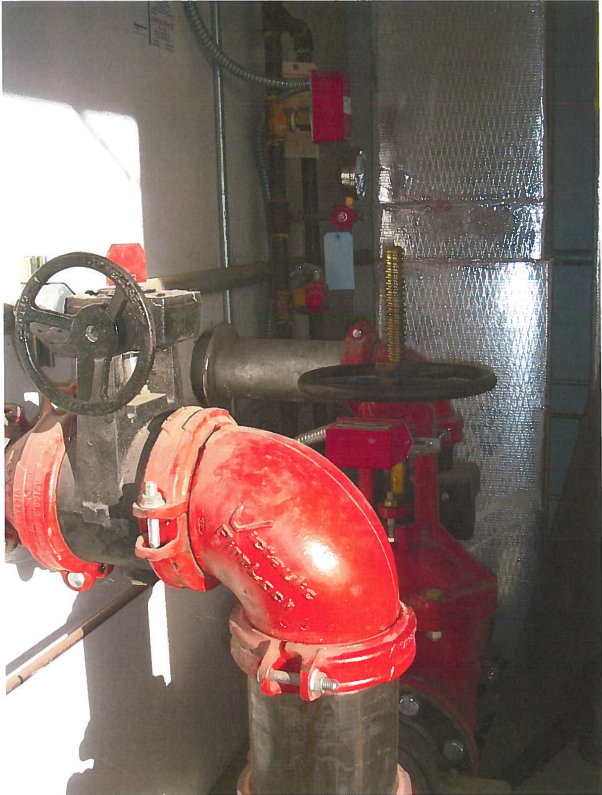
63-31131 License Exam 10/22/2010 Photo #2: Valves and pipes from well discharge pipe (at very bottom of this photo) to outside fire hose hookups.
